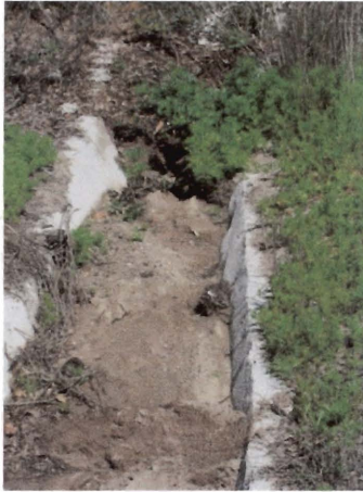
Inadequate maintenance of site drainage.
