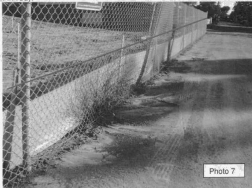
Photo 7: This is the same fence line (in red) shown in Photo 6. Soil binders and track-up/track-down BMPs failed to secure soil and prevent erosion. This photo shows sediment left the site and was discharged to Starlight Drive. This sediment still had not been cleaned up at the time of inspection. This silt fence looked new because of how clean it is. It is unknown if a silt fence was there prior to the rain event.
