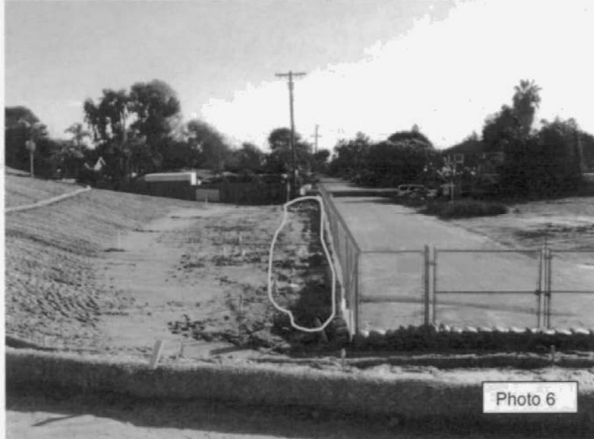
Photo 6: Soil binders were reportedly used in conjunction with "track-up/track-down" BMPs on the slope. These BMPs failed to secure soil and prevent erosion. This photo shows sedimentation at the base of the slope (outlined in yellow) along the fence line (shown in red).
