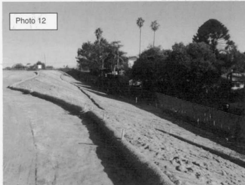
Photo 12: Soil binder plus "track-up/track down" was reportedly used as a sediment control BMP on the slope shown in Photo 12. The fiber rolls in Photo 12 and the gravel bags at the fence line were placed after the rain event and before the inspection because they were free of any sediment and very clean.
