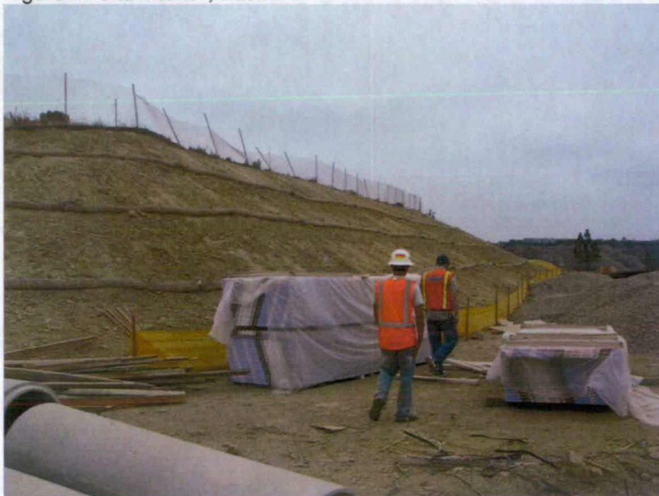
Figure 8. Slope east side; bare soil
