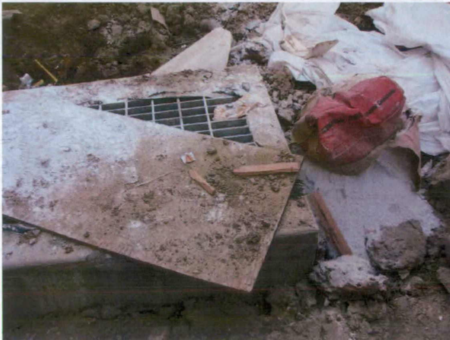
Figure 24. Storm drain littered with construction debris
