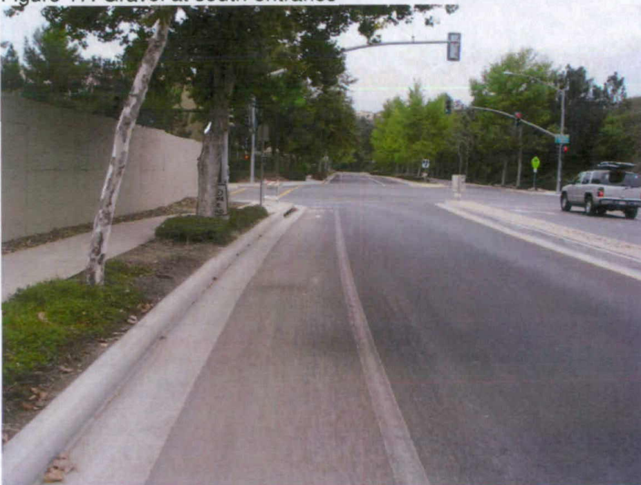
Figure 18. Nearest storm drain downstream; no inlet protection
