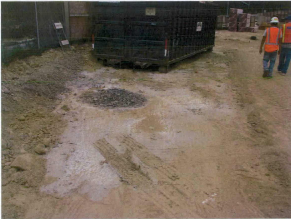
Figure 13. Concrete washout with no containment
