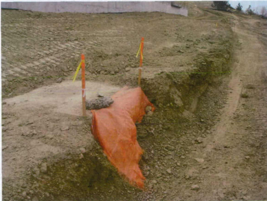
Figure 19. Live storm drain covered with permeable fabric
