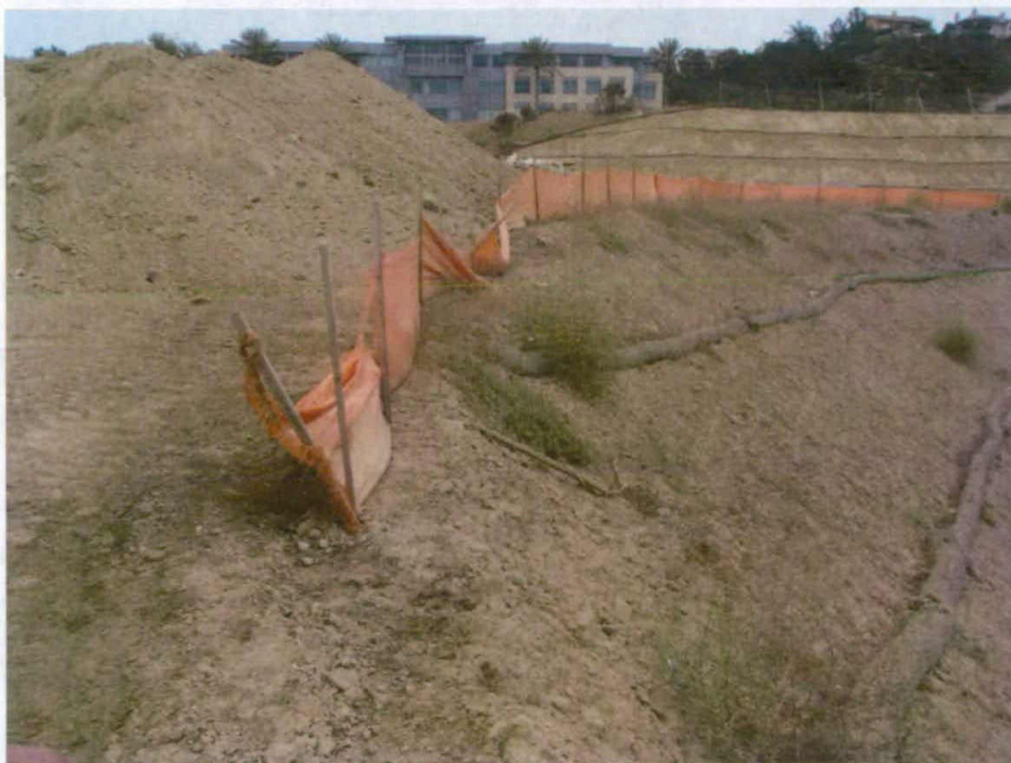
Figure 9. Sediment stockpile with broken silt fence
