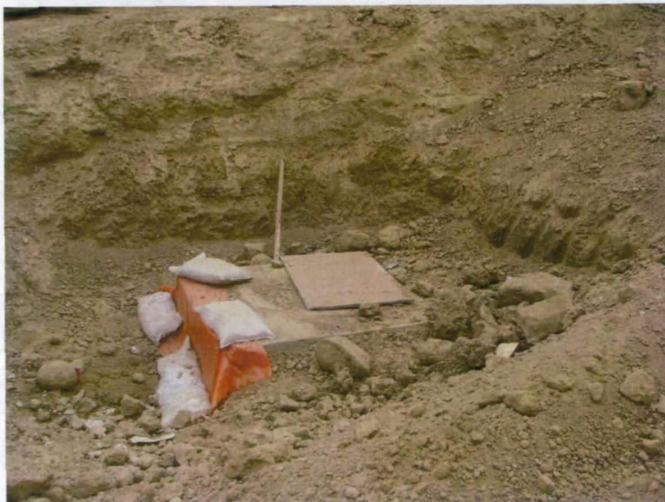
Figure 20. Live storm drain covered with permeable fabric
