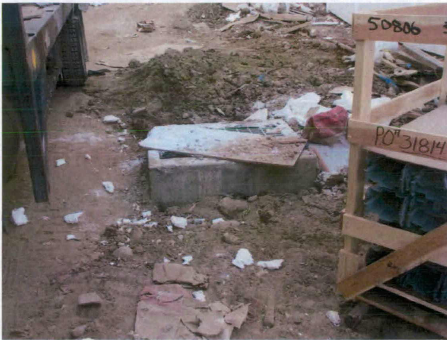
Figure 23. Storm drain littered with construction debris
