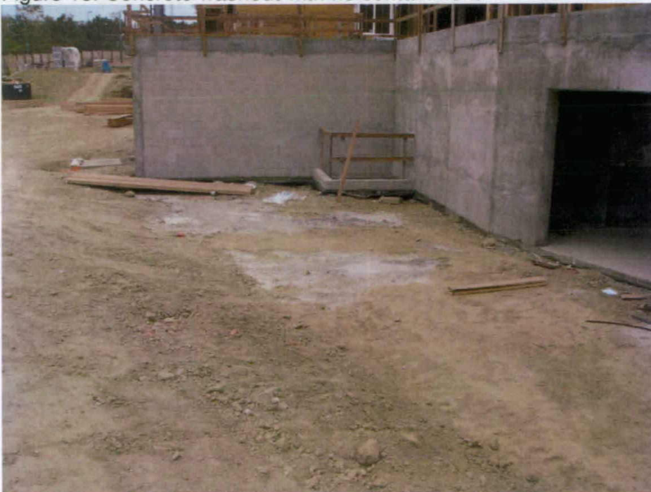
Figure 14. Concrete washout with no containment
