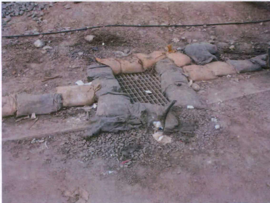
Figure 22. Broken gravel bags
