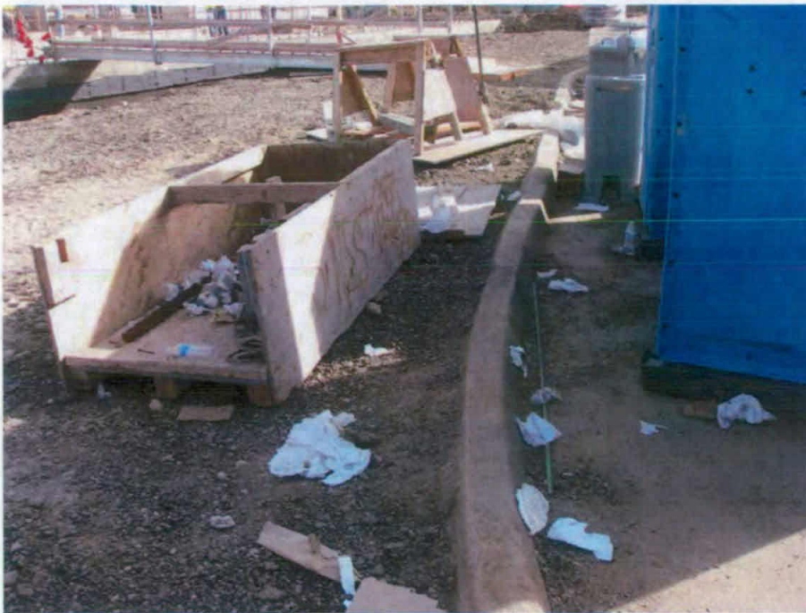
Figure 3. Site interior; trash
