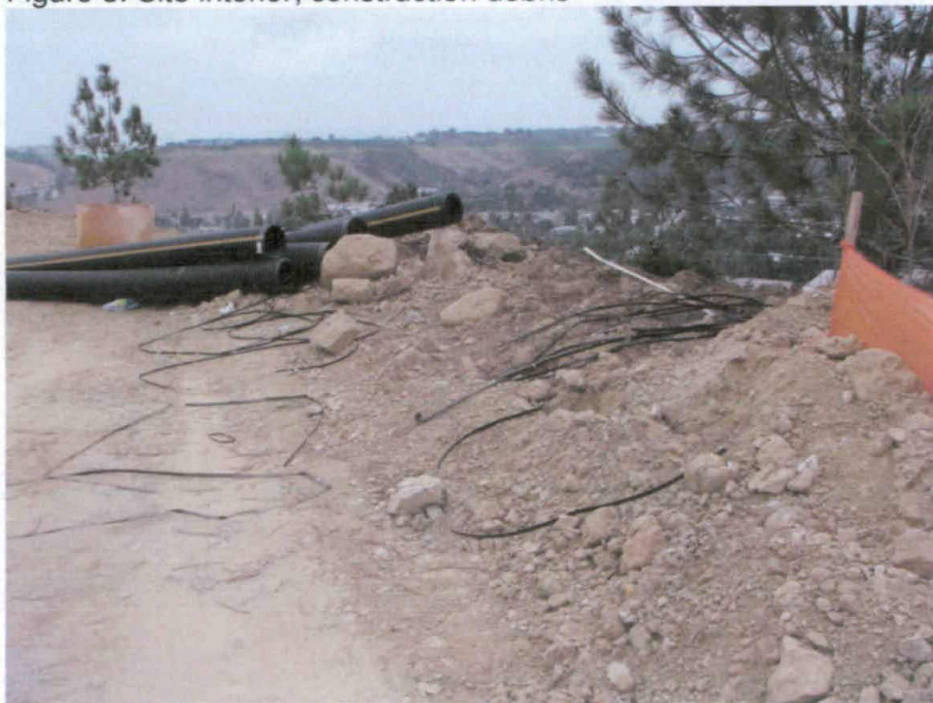
Figure 4. South west side; construction debris
