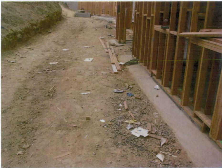
Figure 7. Site interior; trash
