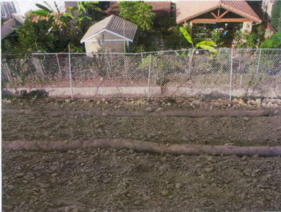
Figure 13. Damaged silt fence
