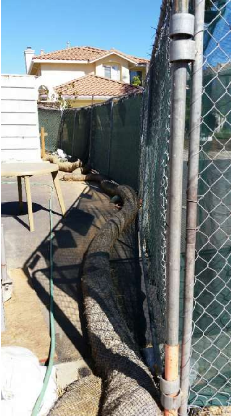
Sediment discharge onto asphalt and improperly installed perimeter control (fiber rolls).
