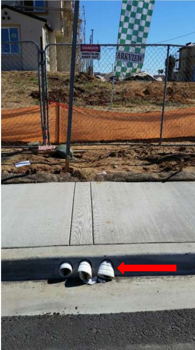
Curb core drains containing sediment.
