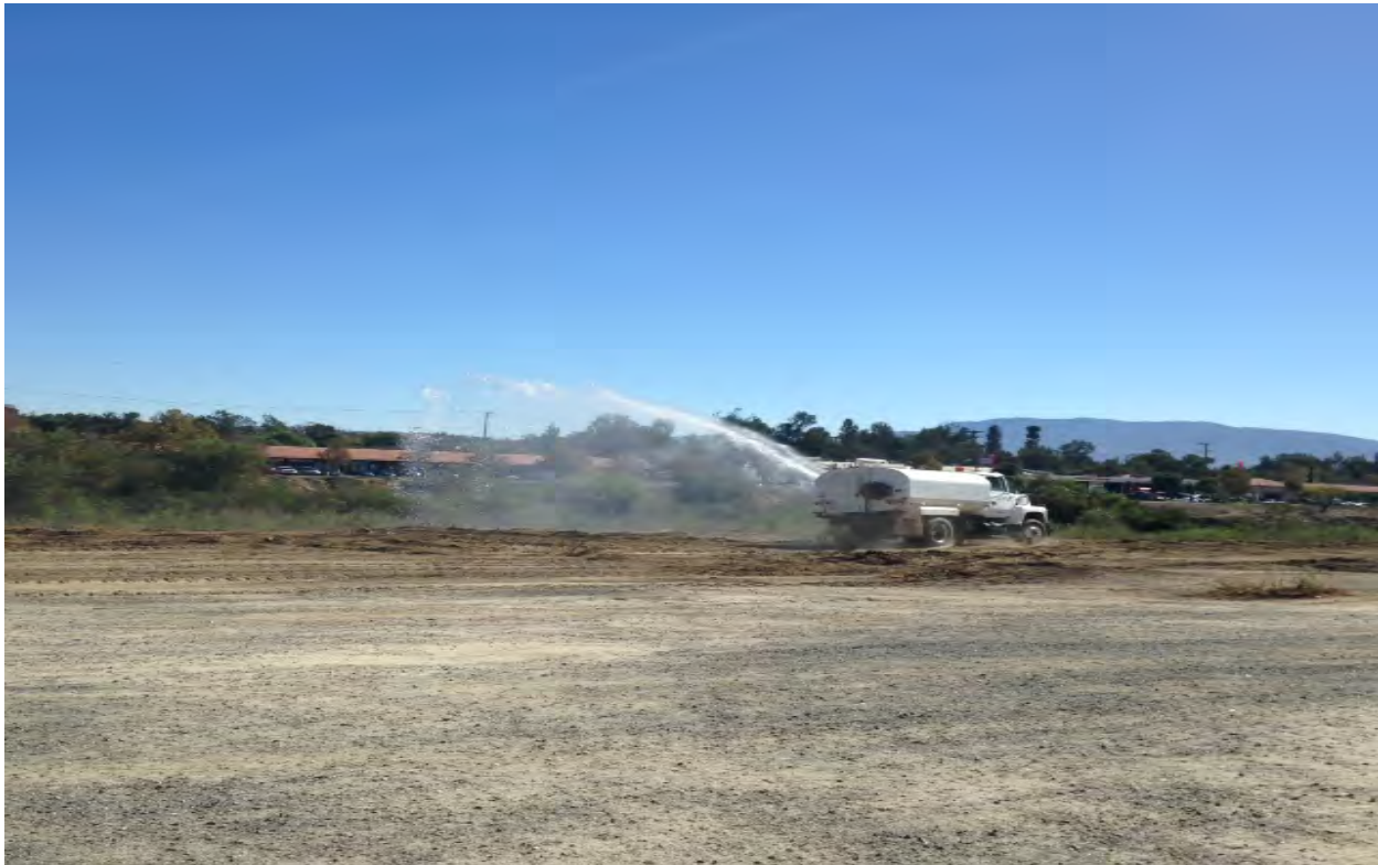
Dust Control: Fulltime Water trucks (2-3 each 4,000Gal Capacity) are being used to keep dust down.
