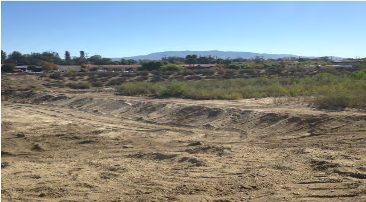
Earthen Berm: 4' Tall X 12' Wide X Bank to Bank Berm placed at the Downstream End of project for Run-off Control.
