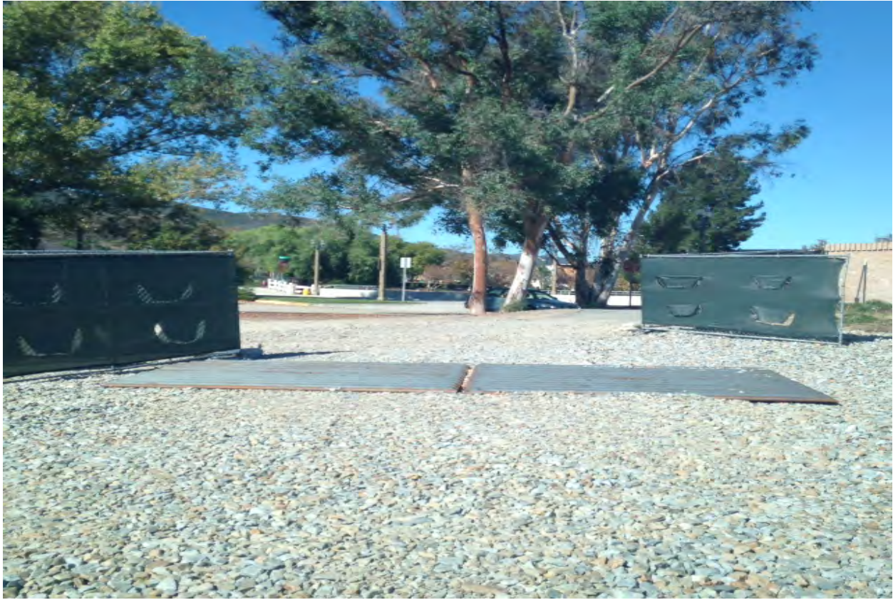
Construction Entrance: Picture of one of our exits (currently not being used) at the south end of project
