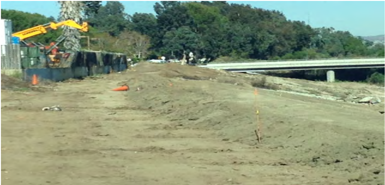
Earthen berms are placed on top of embankments in non-active parts of the creek as part of the run-on protection. North end of the project near Rancho California Rd. This portion of the project from Sta. 107+00 to 102+00 is to be cleared only. OHL has requested US Army Corp to review the current condition and provide contour grading plans as well as any recommended BMPs.
