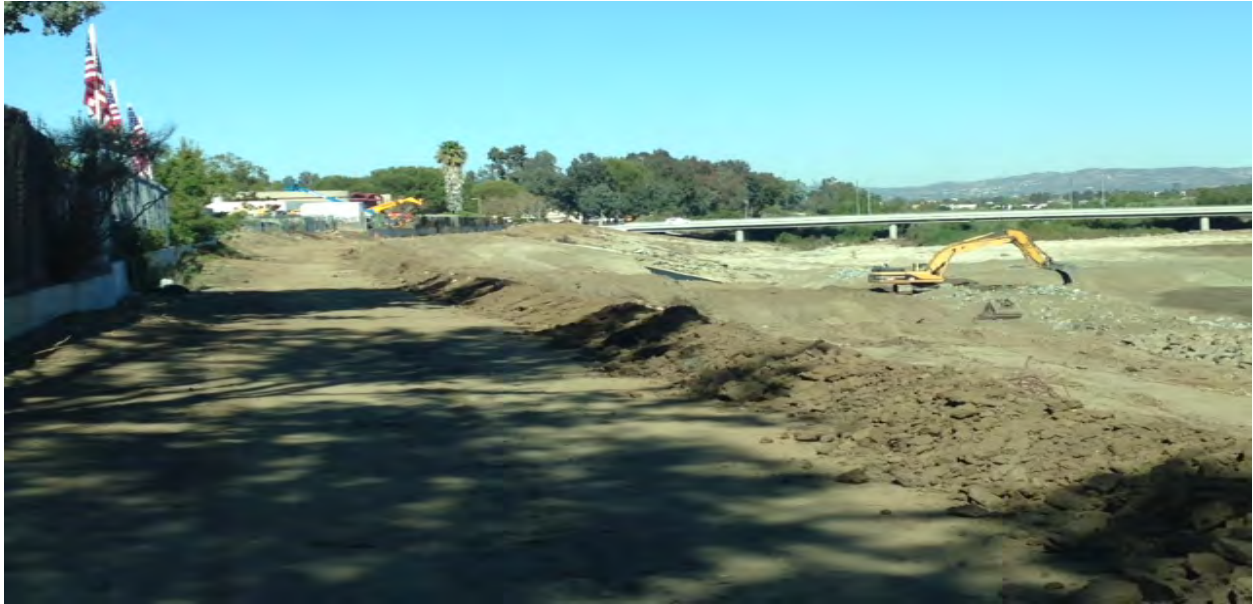
Picture shows riprap being installed as part of the permanent slope protection from Sta. 102+00 to 98+00. The earthen berm on top along the access road is a part of the temp. run-on control.
