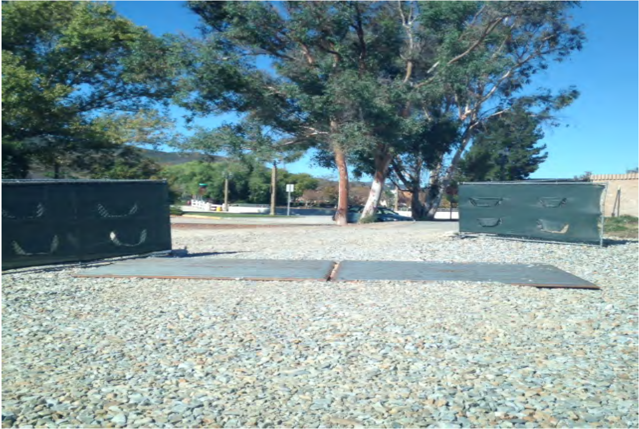
Construction Entrance: Picture of one of our exits (currently not being used) at the south end of project
