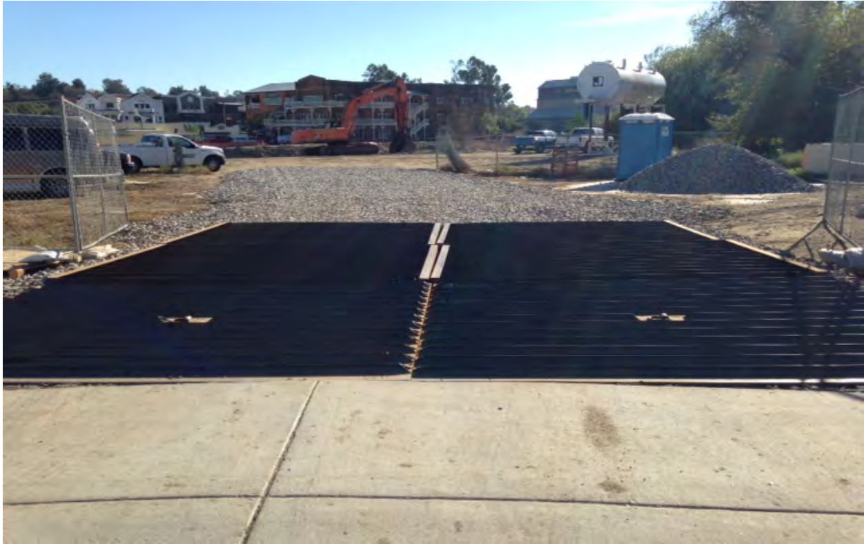
Main construction entrance near Felix Valdez Rd. (90def bend). Rock and track-out plates are cleaned and maintained daily or as needed.
