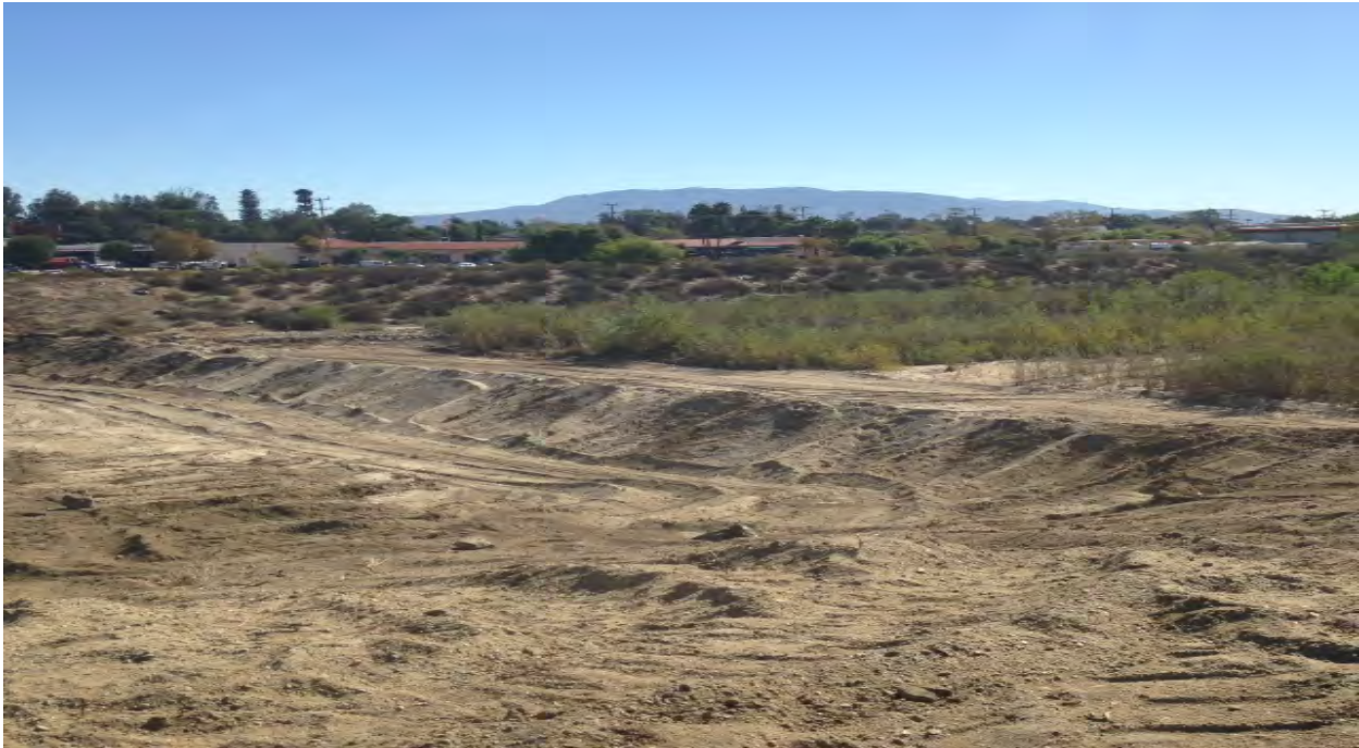
Earthen Berm: 4' Tall X 12' Wide X Bank to Bank Berm placed at the Downstream End of project for Run-off Control.
