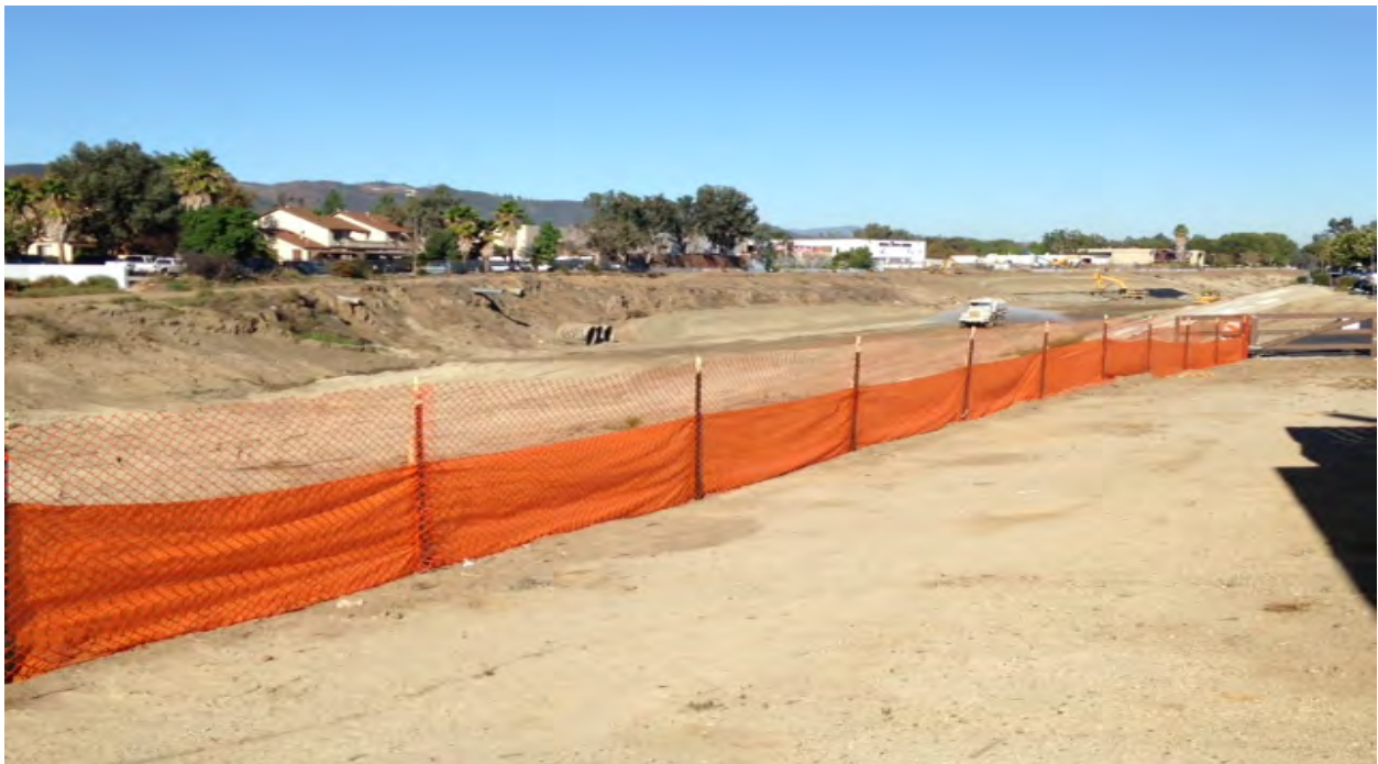
This is along the eastside of the creek approx. 1,500 ft downstream of the Rancho California Rd. OC. Silt fence is in place as part of the run-on control.
