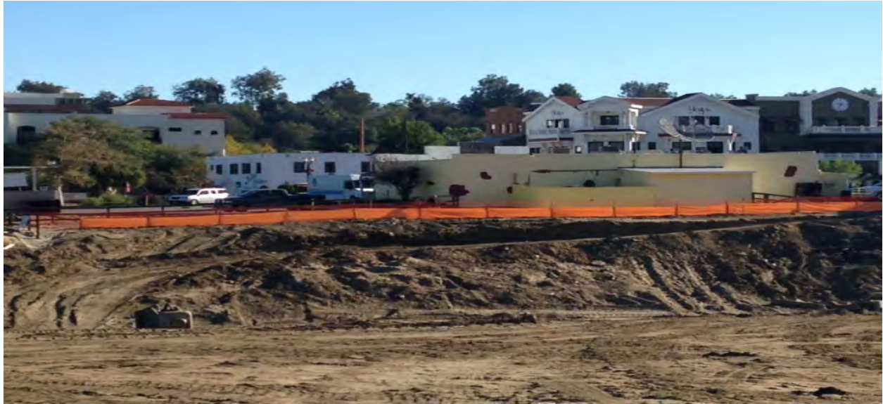
Eastside bank at Approx. Sta. 84+00 to 78+00. Silt fence in place for run-on control.
