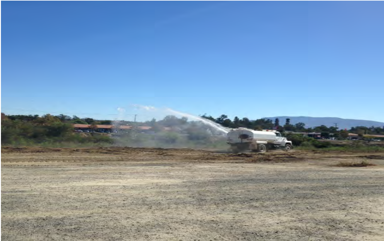
Dust Control: Fulltime Water trucks (2-3 each 4,000Gal Capacity) are being used to keep dust down.
