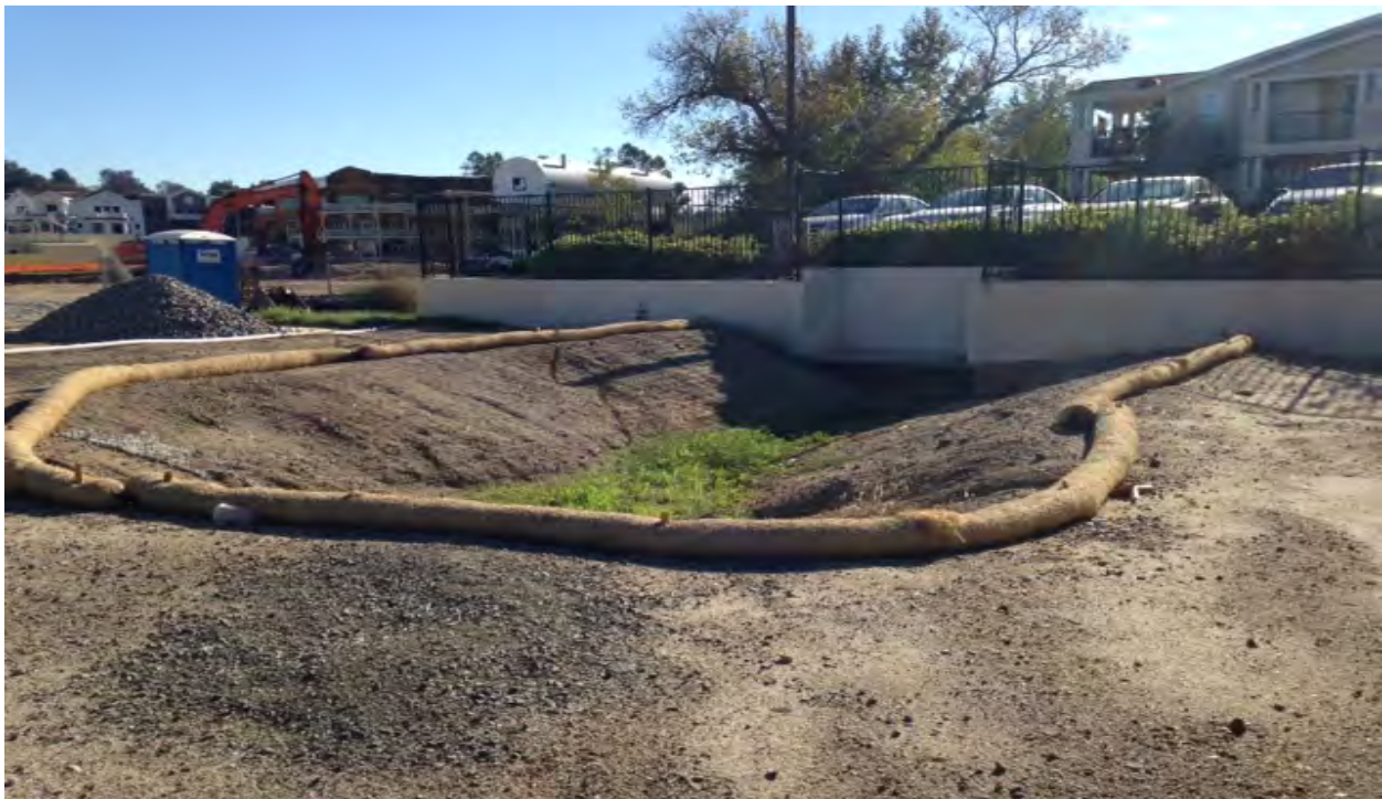
Earthen swale near Felix Valdez road is protected using fiber rolls as perimeter control.
