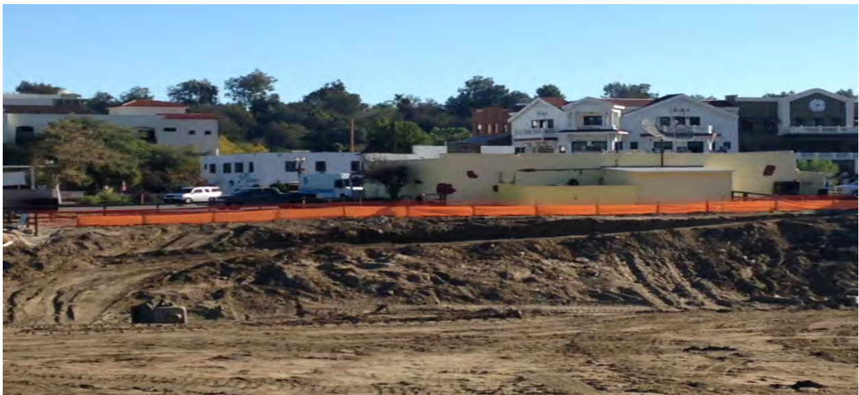
Eastside bank at Approx. Sta. 84+00 to 78+00. Silt fence in place for run-on control.
