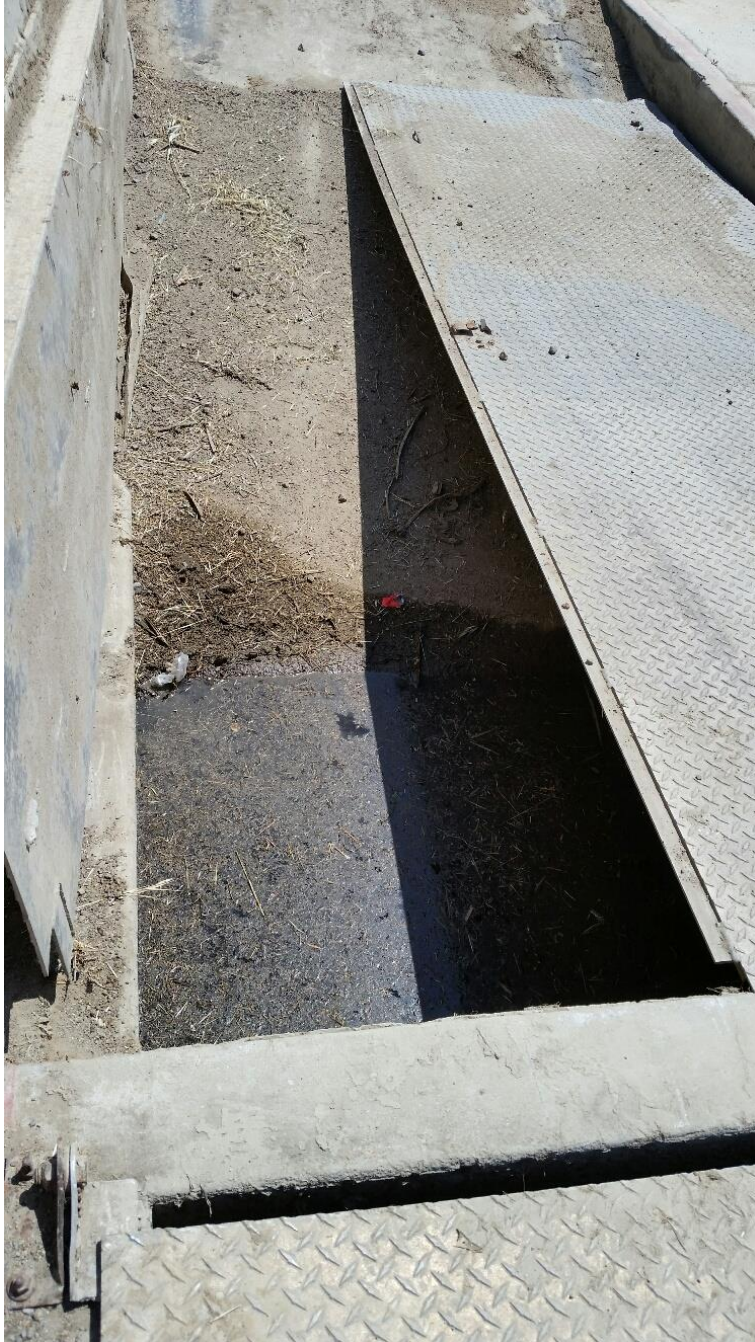
Photo #41- Standing water in vault sump.
