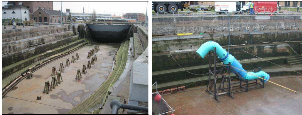
figure 2.1 Dry dock 'Jan Blanken' (left) and pump in dock (right).
