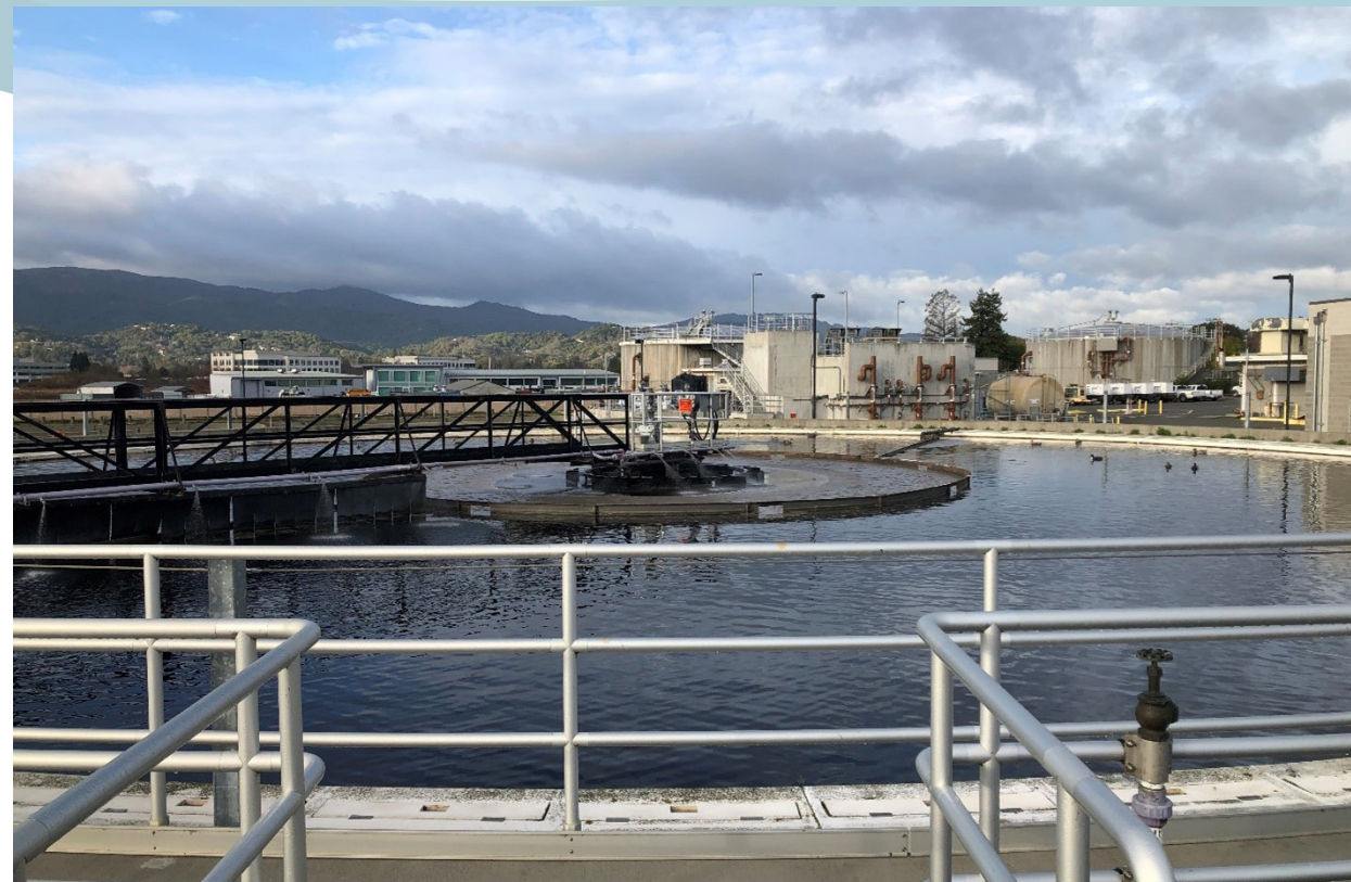
Photo to left: Secondary clarifier at Novato Sanitary District's wastewater treatment plant, covered under a NPDES permit
