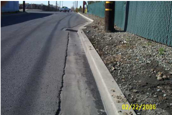
Sediment in curb just outside the facility fence
