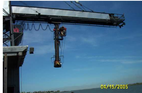
Loading chute is lowered directly into hold of the ship to reduce dust emissions
