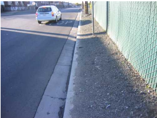
Sediment in curb just outside the facility fence
