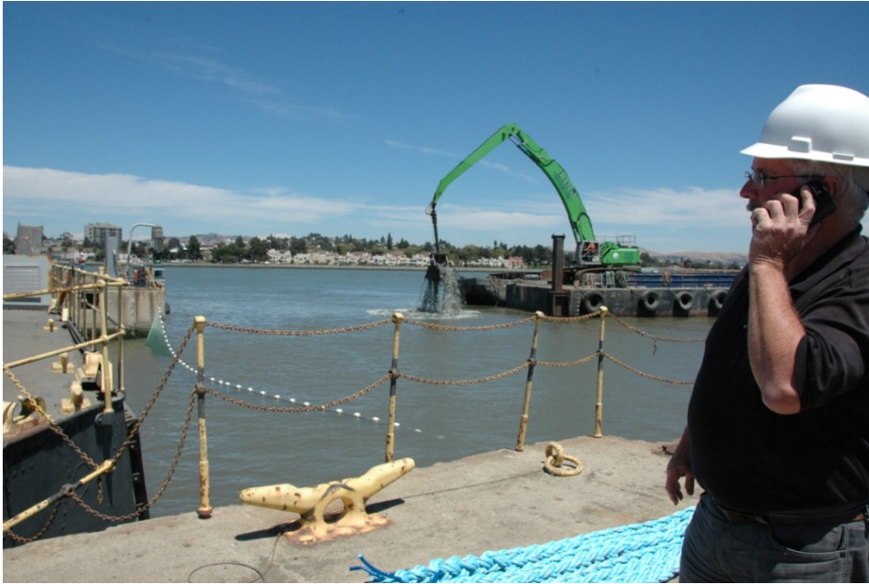
Photo 1a. Dredging the approach to Dry Dock 3 at Mare Island Ship Yard.
