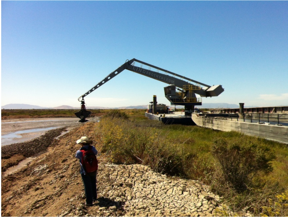
Photo 1c. Offloader placing dredged material on inboard side of levee at Cullinan Ranch.
