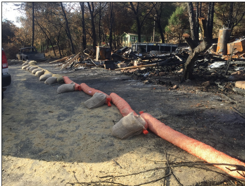
Figure 1. Perimeter controls installed around burnt structures and debris in the Sonoma Creek Watershed
