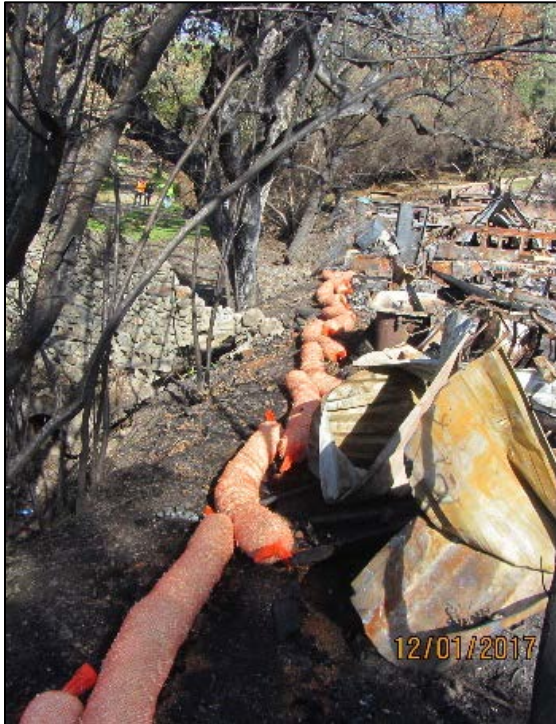
Figure 6. Erosion and drainage controls installed next to burned structure near Sonoma Creek.
