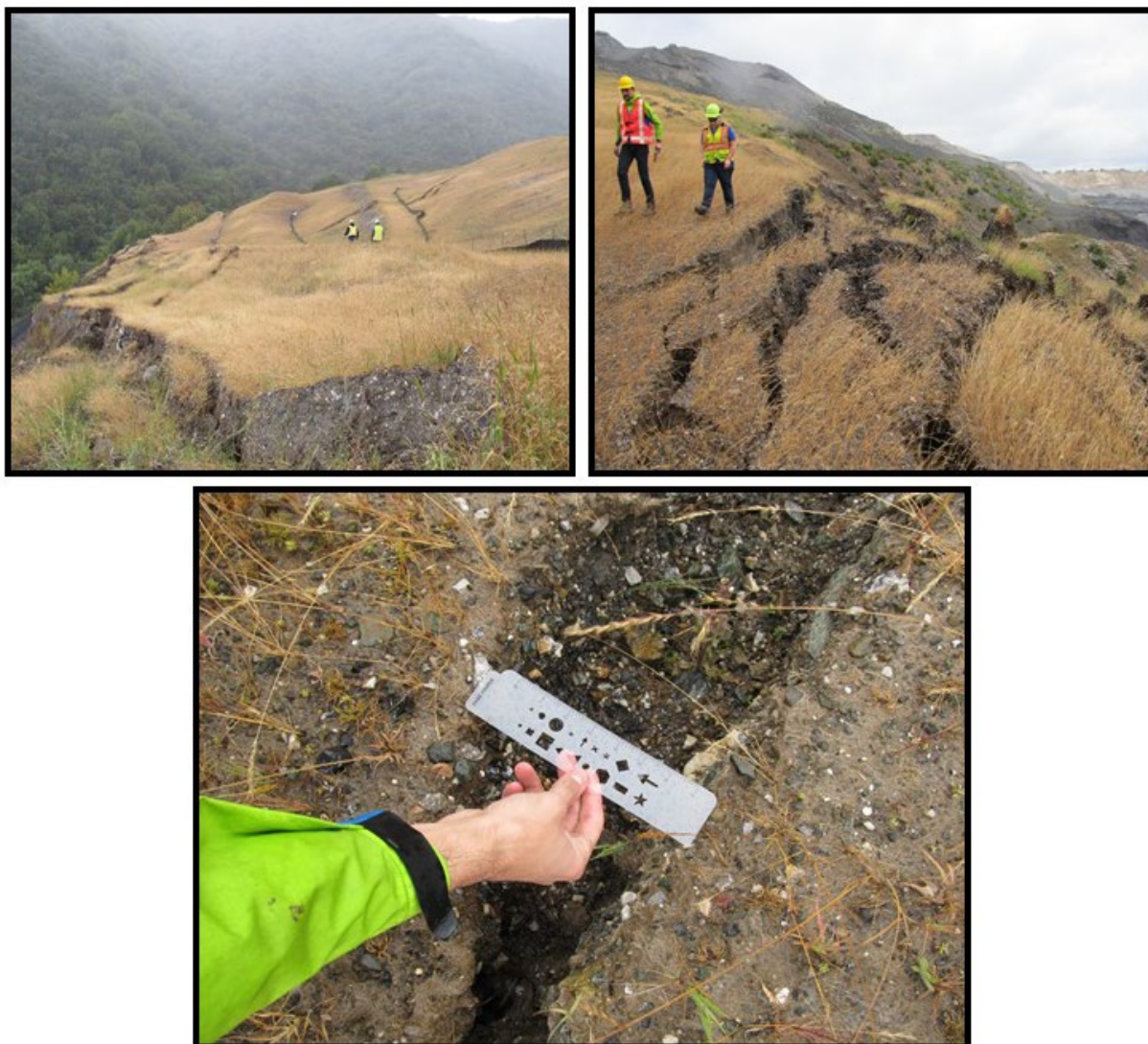
Figure 2. Cracks and fissures on slope above Permanente Creek.
