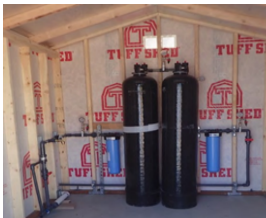
New Ion Exchange Filtration System
