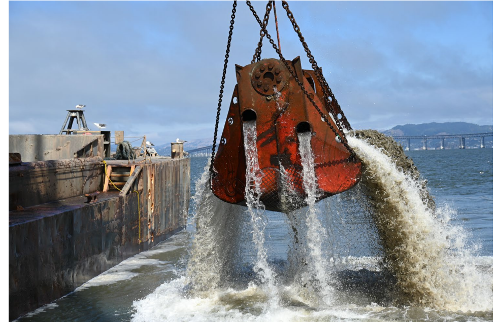
Photo of a clamshell dredge coming up from the bottom of Richmond Harbor during maintenance dredging.
