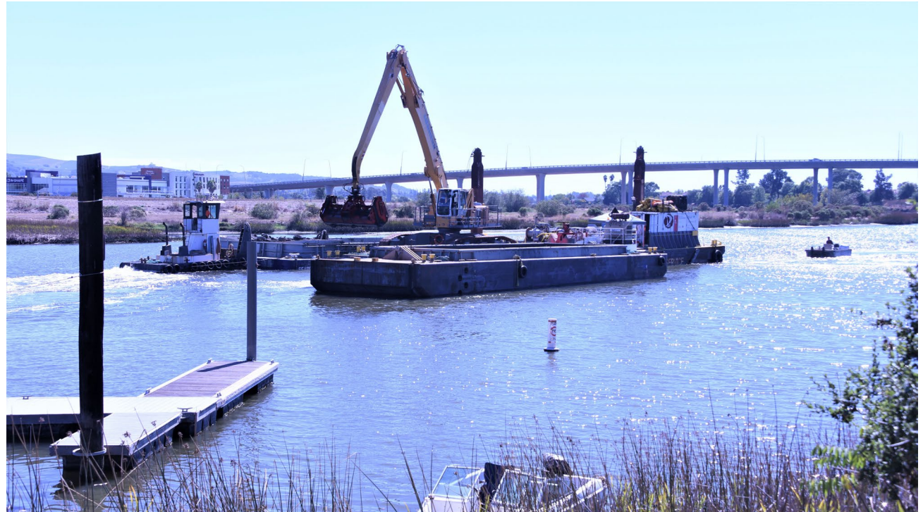
Photo of maintenance dredging in the upper portion of the Napa River.
