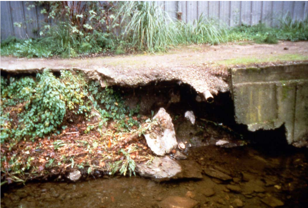
Figure 16B. Before Project Conditions: Concrete failure
