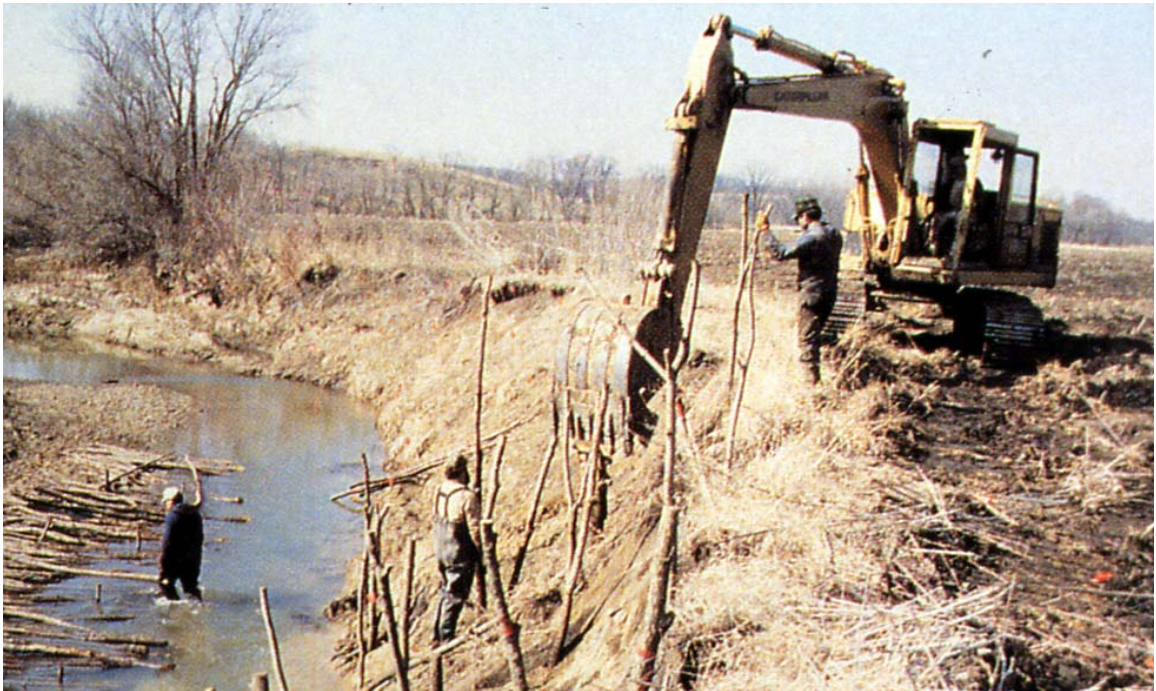
13 D Photo: Mechanical installation of willow or cottonwood posts. Illinois Water Survey
