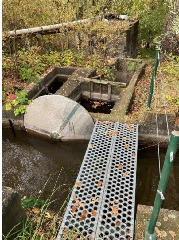
Turnout from Orwick Ditch onto former Tompkins Ranch lands.
