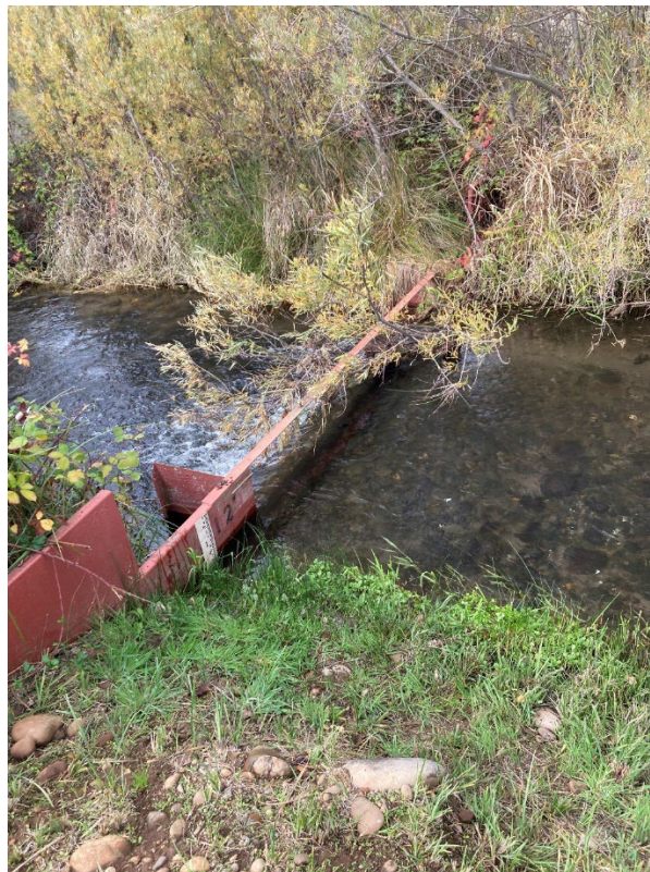
Orwick Ditch rectangular measurement weir, facing west.
