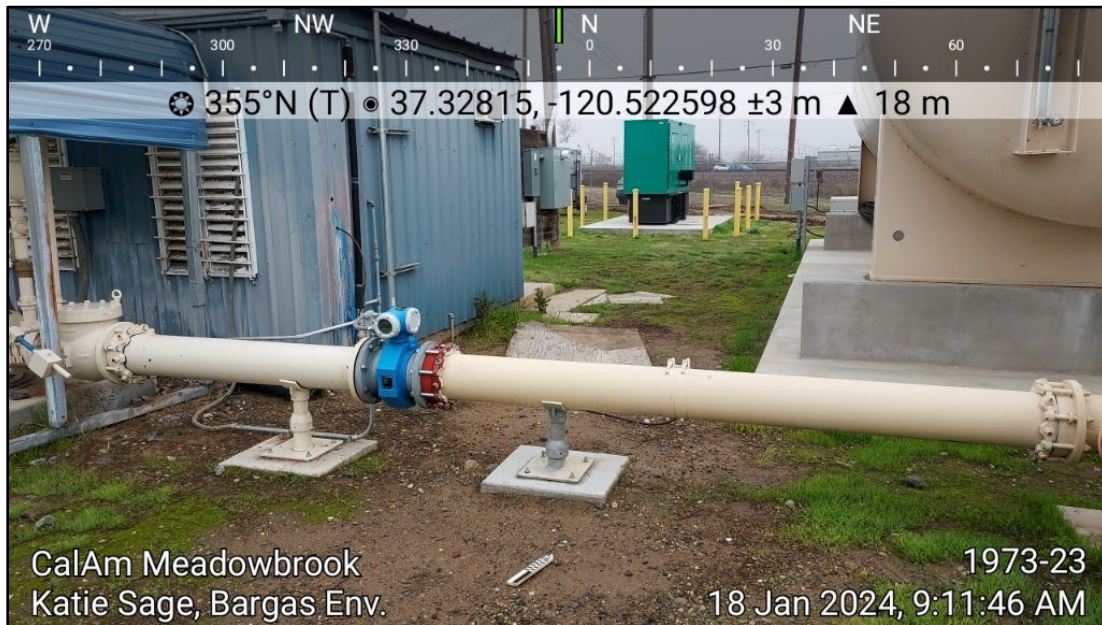
Figure 8. Standing pump structures within gated pump area (Project Area). View toward the North.
