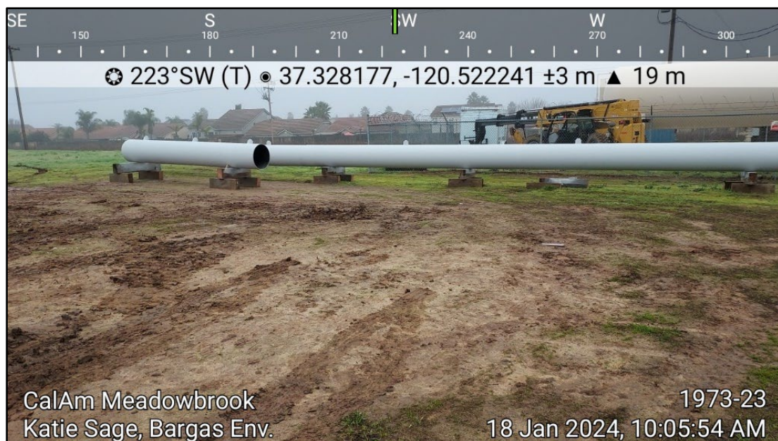
Figure 10. Graded bare area, east of gated pump area. View toward the Southwest.
