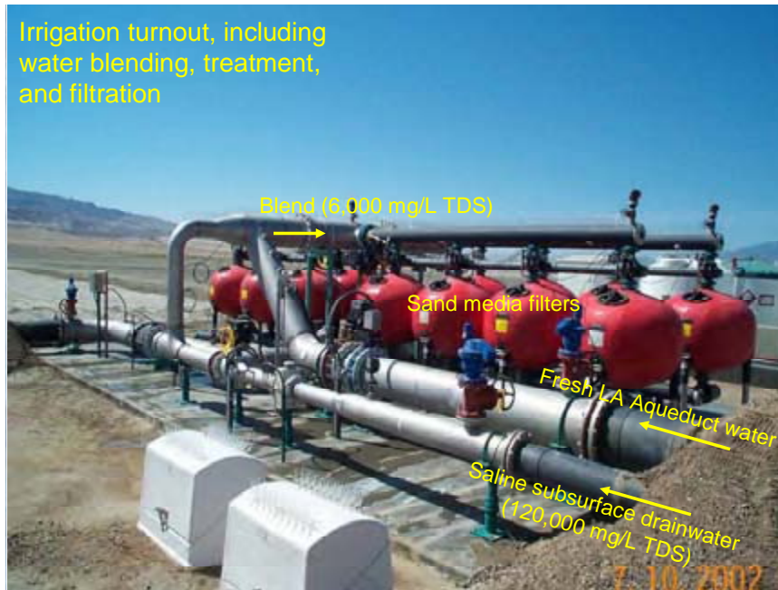
FIGURE B6 Blending and filtration facilities at turnout from main pipeline.
