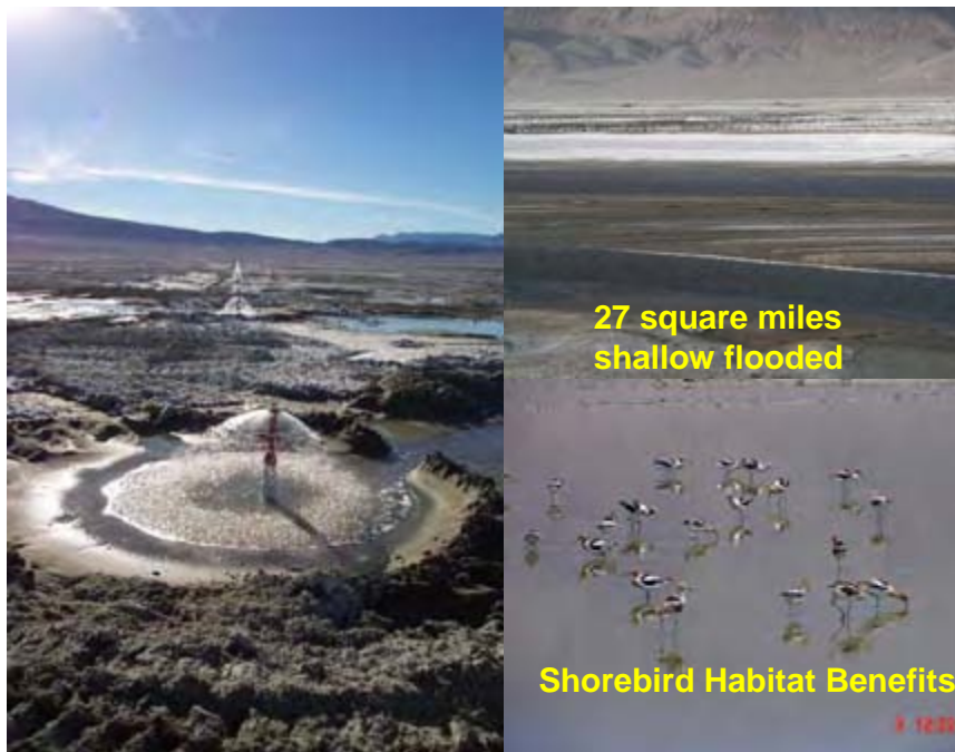
FIGURE B14 Views of shallow flooding facilities at Owens Lake.
