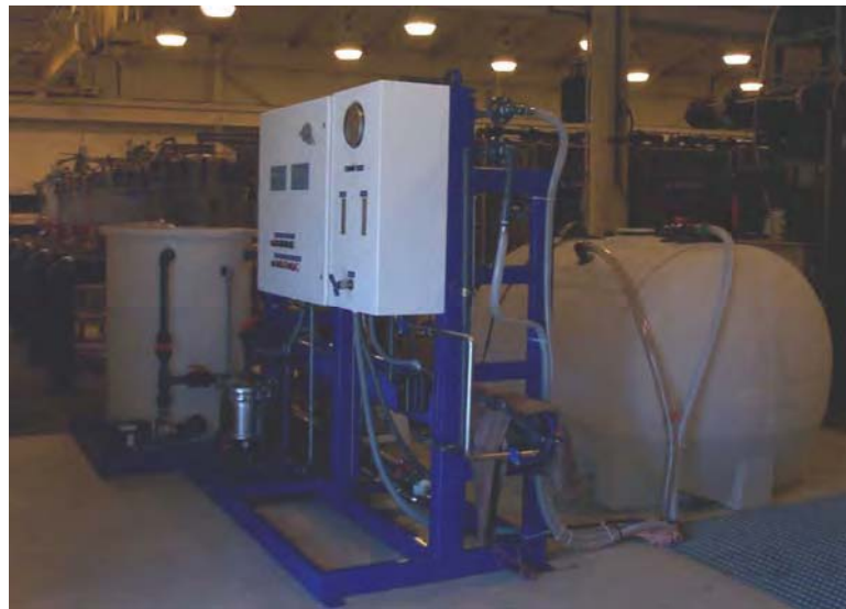
FIGURE F2 Photo of the MWD GrahamTek RO System
