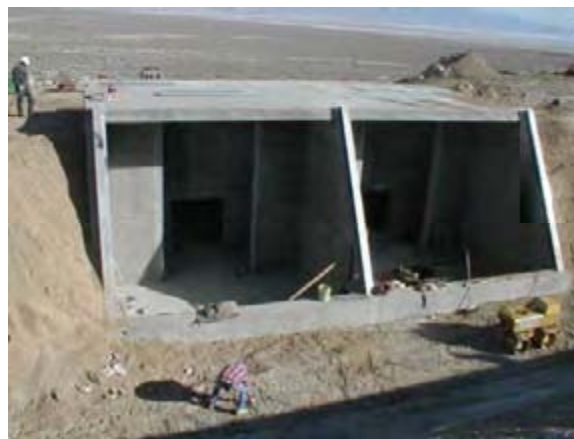
FIGURE B10 One of two diversions in the Los Angeles Aqueduct supplying freshwater to the Playa. Downstream of these points, water is conveyed and distributed in pipes ranging from less than 1 inch to 60 inches in diameter.
