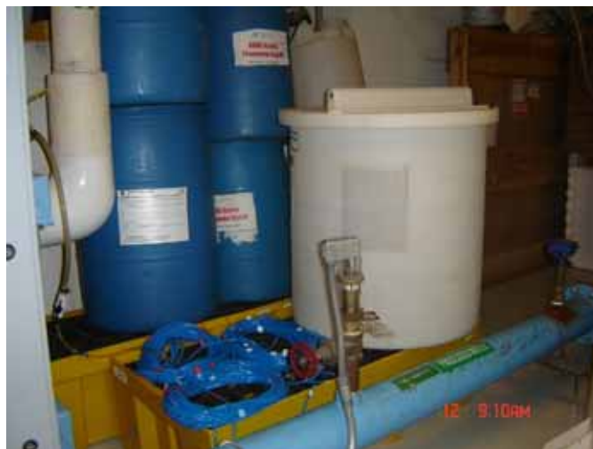
Figure 7.13. The three coiled branches of the pipe loop installed at the NY location. Each branch is 150 ft long and has a flow rate of 1.54 mL/s. The loop branches are color-coded in increments of 5 ft to permit easy identification of the sampling points.
