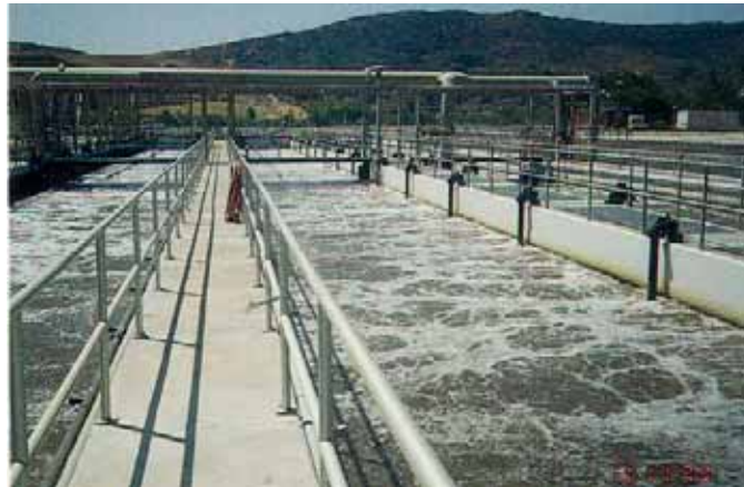
Figure 3.4. An activated sludge aeration lane.
