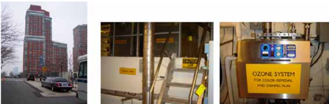
Figure 7.5. A high-rise apartment in NY that meets all its toilet and landscaping needs with reclaimed water. The treatment plant is located in the basement (center), and the finished water is disinfected with UV/ozone treatment.
