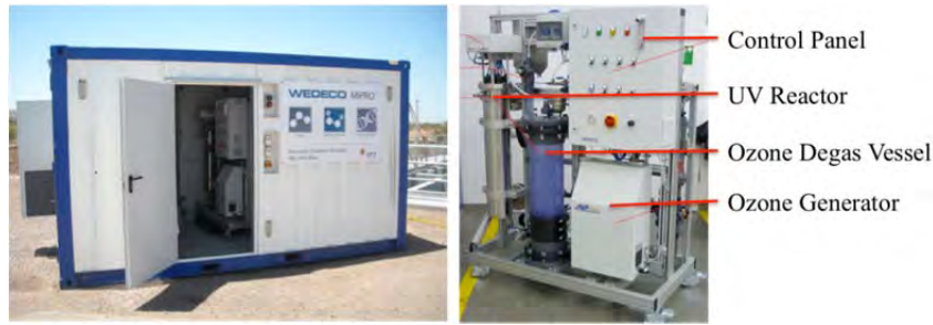
Figure 6.10. Green Valley Water Reclamation Facility pilot.
