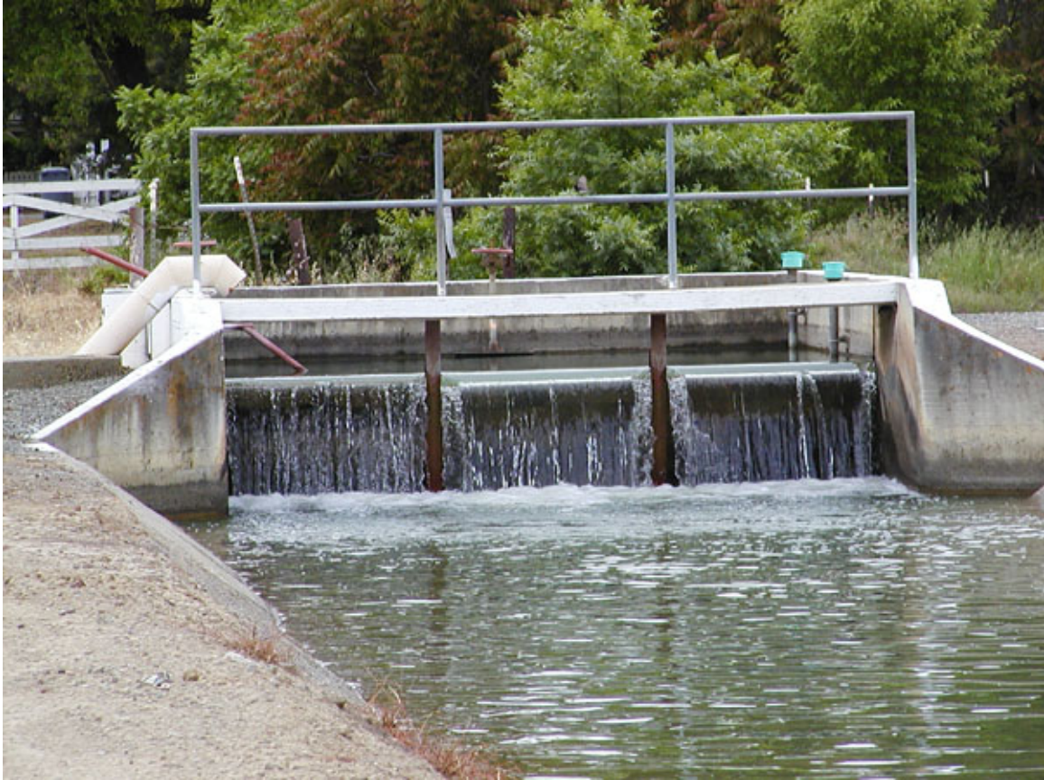
Figure 5. Byrnes Canal Weir A under low flow conditions on May 1 st 2003. Site of normal applications.
