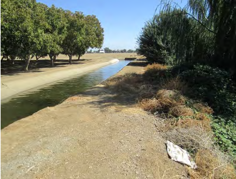
Photo 3. 45 Canal where it runs just north of Kellogg Creek within BBID, looking east.
