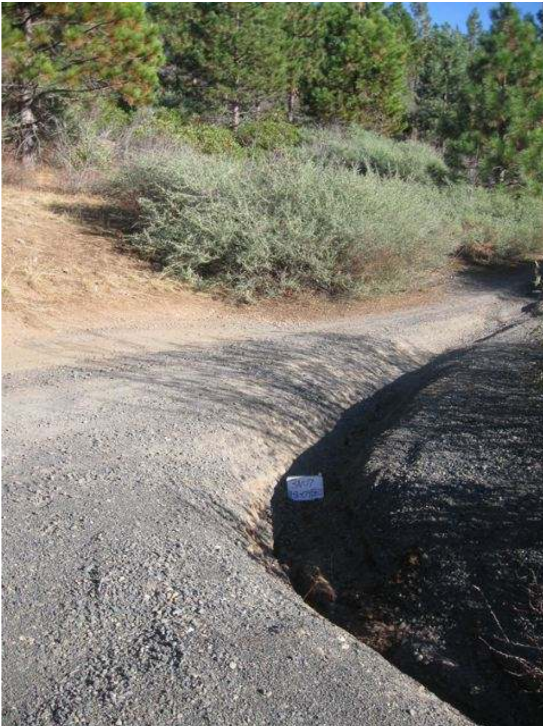
This road rut diverts sediment-laden water from Forest Road 3N86 into Hull Creek.
