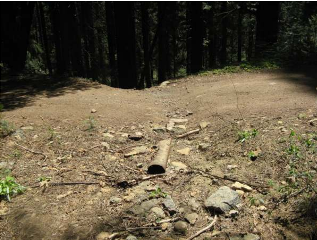
Failed culverts are common. This failed culvert results in sediment to creek at top of photo.
