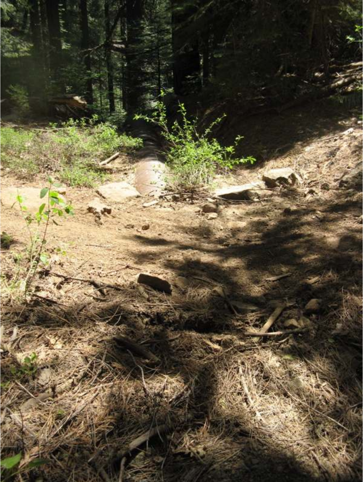
Another failed culver, this one on a motorcycle trail.
