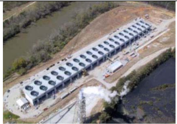
Retrofit 40-cell back-to-back inline conventional cooling tower, coal-fired Plant Yates (GA) – 40 cells is adequate size for up to 1,100 MW nuclear reactor.
