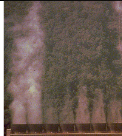
Effect of plume abatement function – Plume abatement off, left two cells. Plume abatement 100% on, adjacent two cells. Source: P. Lindahl – Marley presentation, May 2002.
