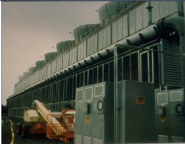
Operational plume-abated tower, ~60 ft. tall – Selkirk 2 Cogen, 330 MW (NY) Source: P. Lindahl – Marley presentation, May 2002.
