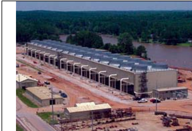
36-cell, space saving back-to-back inline conventional cooling tower. From: GEA Power Cooling Systems website
