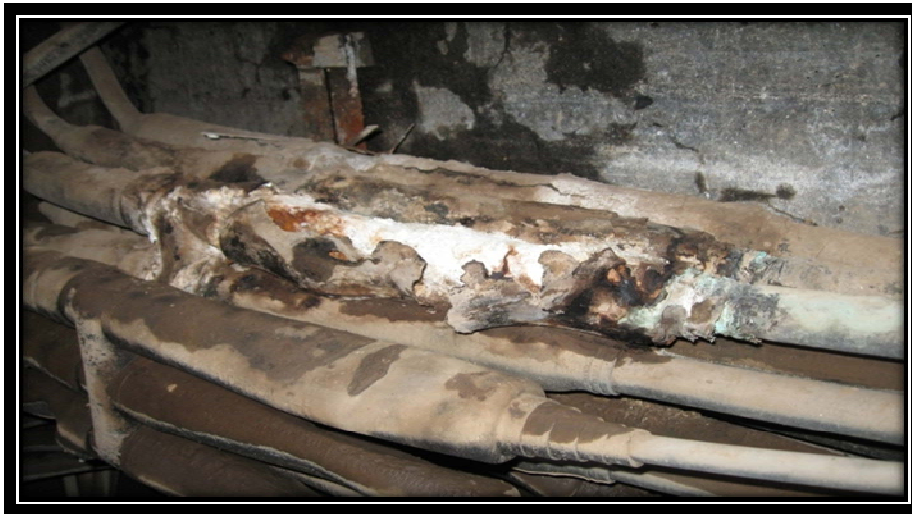
Picture: Illustrative of Cable Scheduled for Replacement.
