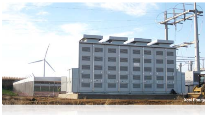
Figure K-3. Sodium-sulfur batteries.
