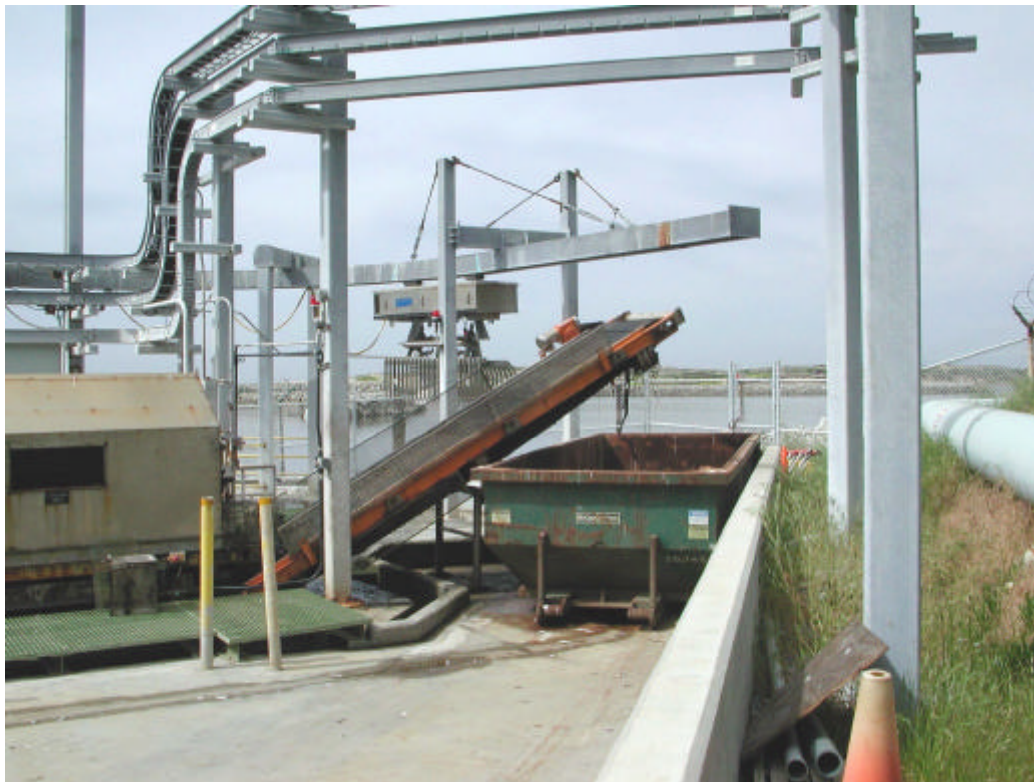
Figure 2-6. Traveling water screen debris conveyor system. Bar rack rake is in the background.
