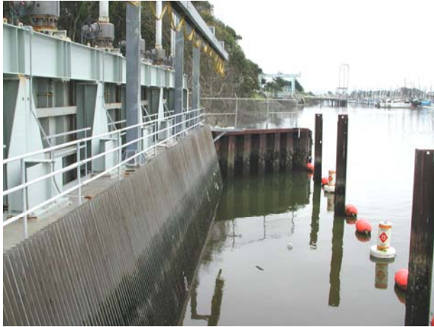
Figure 2-3. Units 1&2 intake bar racks.
