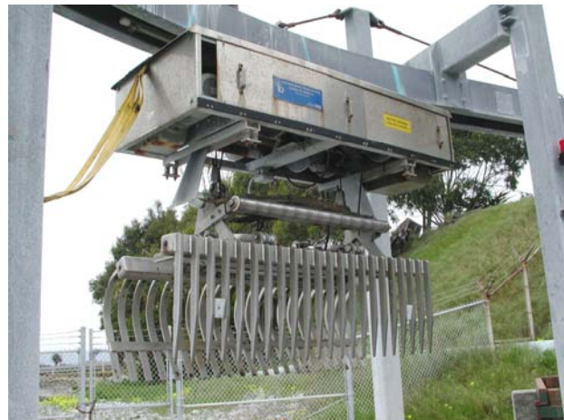
Figure 2-4. Units 1&2 intake bar rack rake.
