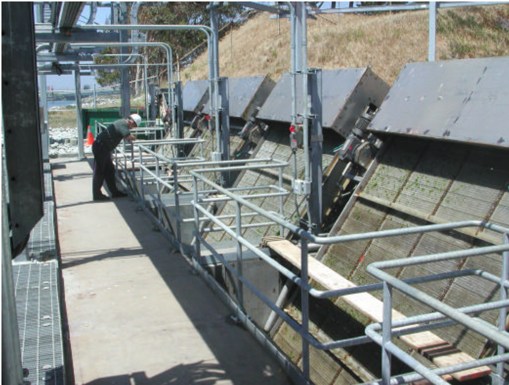
Figure 2-5. Units 1&2 traveling water screens. Four of the six screens are shown.
