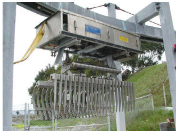
Figure 2-4. Units 1&2 intake bar rack rake.
