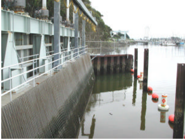
Figure 2-3. Units 1&2 intake bar racks.
