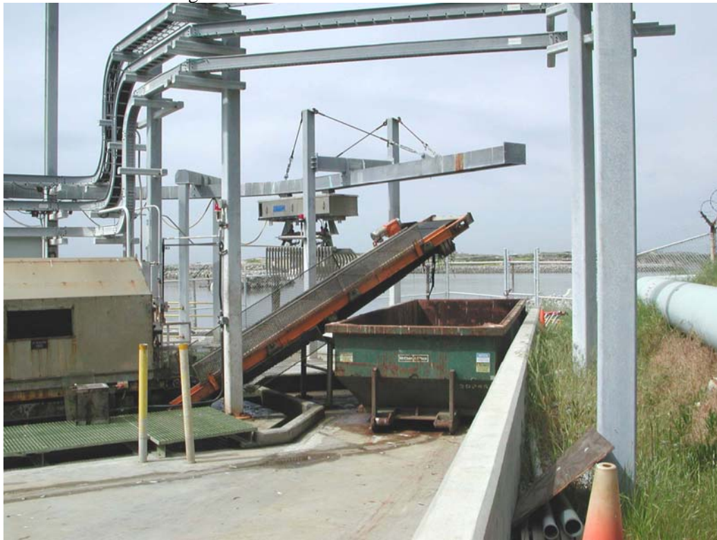
Figure 2-6. Traveling screen debris conveyor system. Bar rack rake is in the background.
