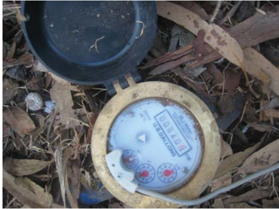
5-1g. Daily Water Metering- Emerald Bay
