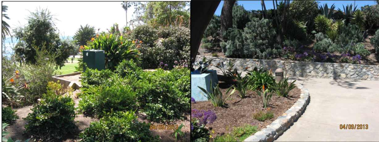
Photos – SmartTimer irrigation controller with antennae on top, water-wise plants in landscaped area.
