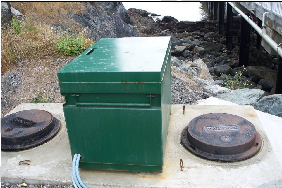
Photo 9. Trinidad Pier, stormwater treatment system housing and percolation wells.
