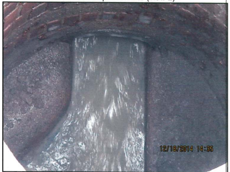
Photo 14: Manhole and sewer line inspection and trunk line on right with high flows
