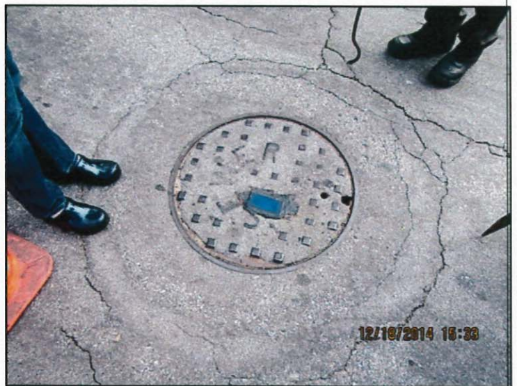
Photo 26: "Smart Cover" inspection site (view 2)
