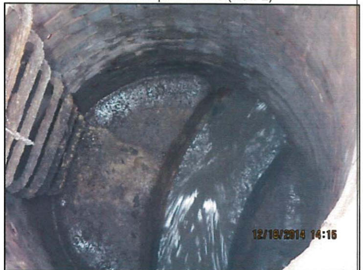
Photo 6: Manhole and sewer line inspection; note LACSD trunk line on right with high flows
