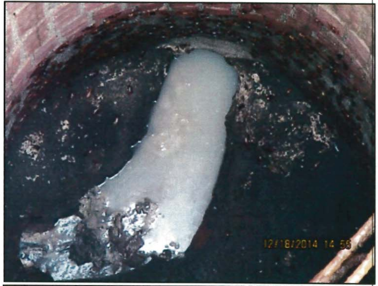
Photo 20: Manhole inspection; note heavy buildup on manhole base and in sewer line
