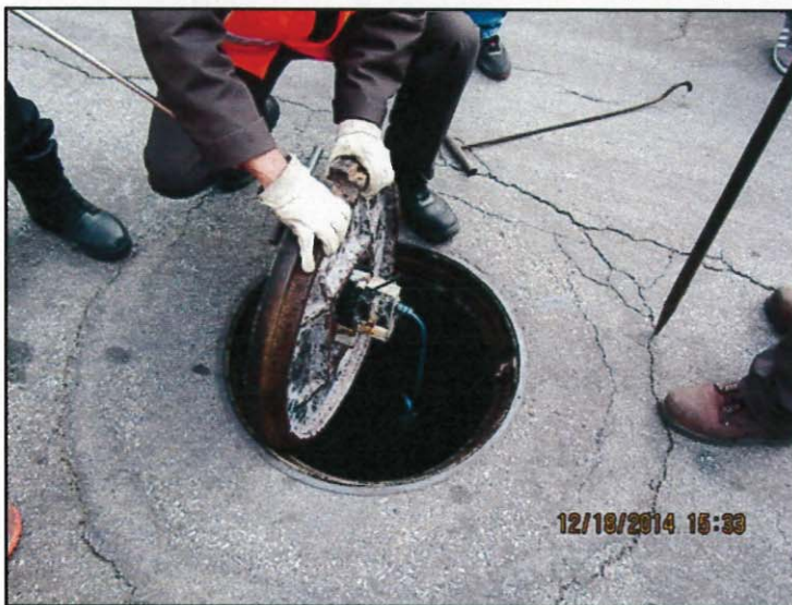
Photo 27: "Smart Cover" inspection site (view 3)
