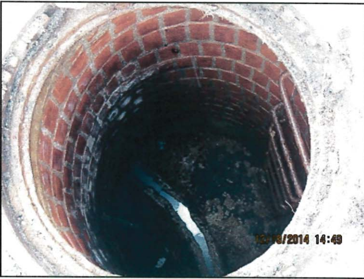
Photo 17: Manhole inspection (view 2): note heavy FOG buildup on manhole base and in sewer line
