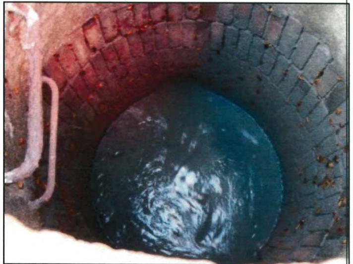
Photo 14: High sewage level with pipe nearly full (view 3)
