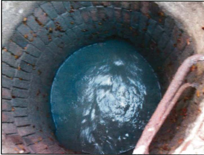
Photo 13: High sewage level with pipe nearly full (view 2)
