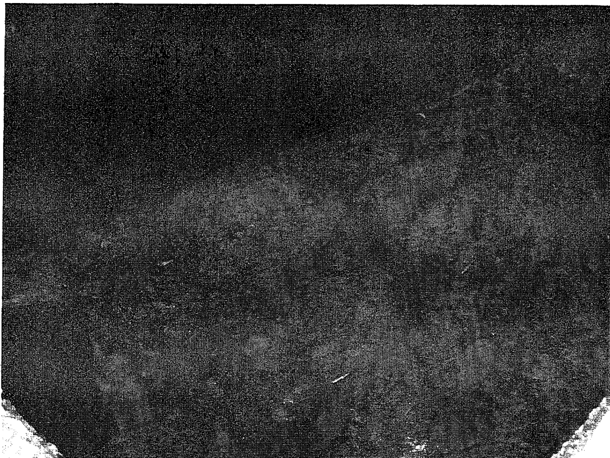
Figure 2: Sewer Plant #7, note the substantial FOG floating on the surface in the wet well. Photograph was taken on December 20, 2011 by Chris Lopez, inspector for the State of California, Los Angeles Regional Water Board.
