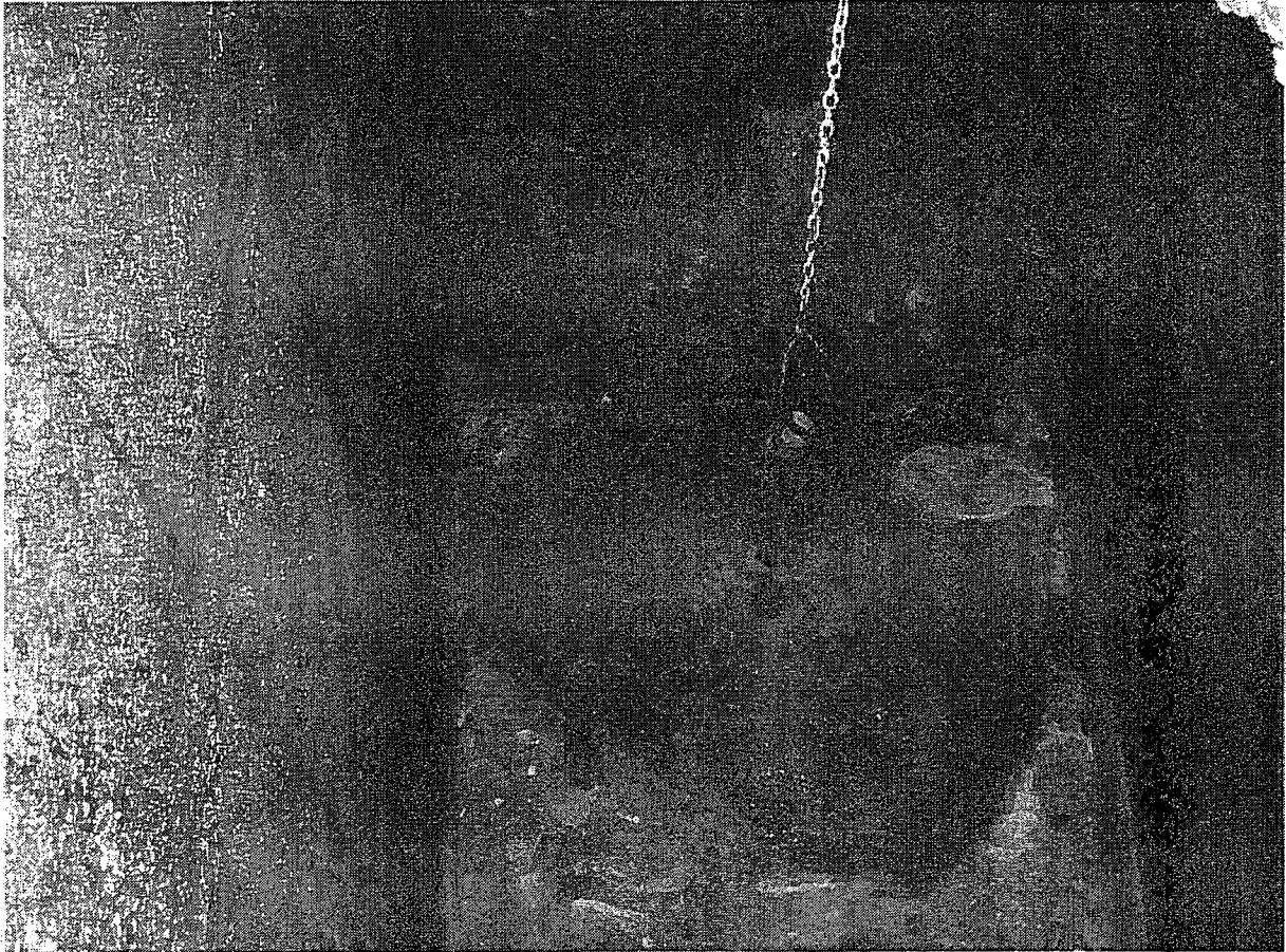
Figure 1: Sewer Plant #7, note the substantial FOG floating on the surface in the wet well. Photograph was taken on December 20, 2011 by Chris Lopez, inspector for the State of California, Los Angeles Regional Water Board.
