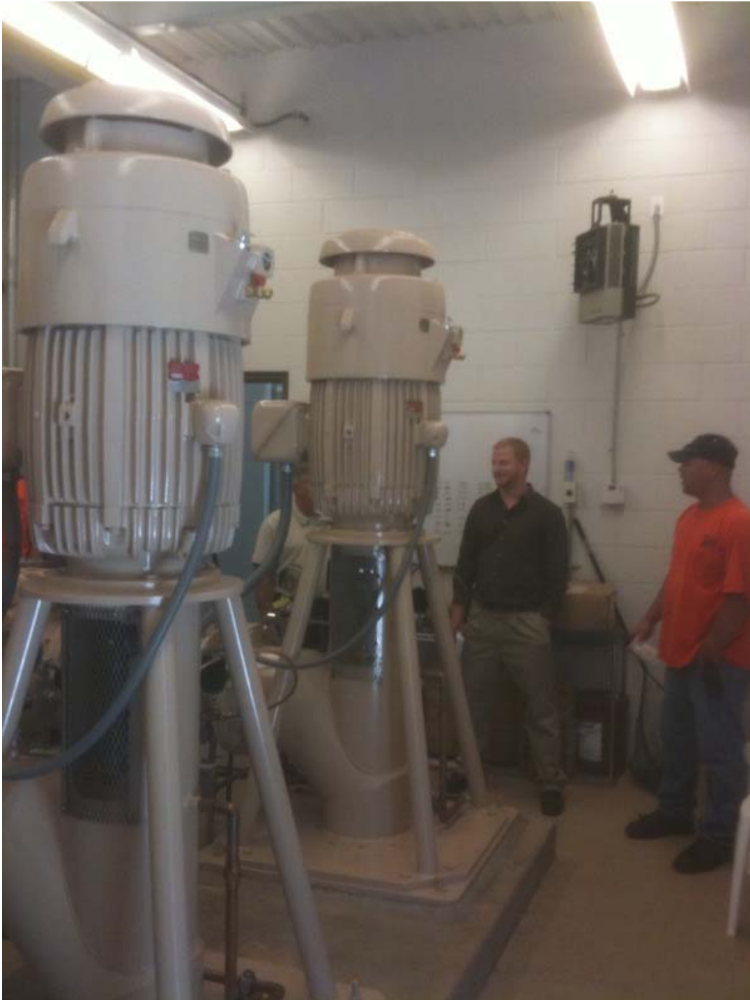
Photo 14: Inspection of North Market lift station including review of inspection and operating procedures for lift station
