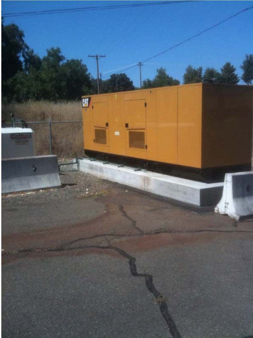
Photo 18: Sunnyhill lift station dedicated emergency backup generator
