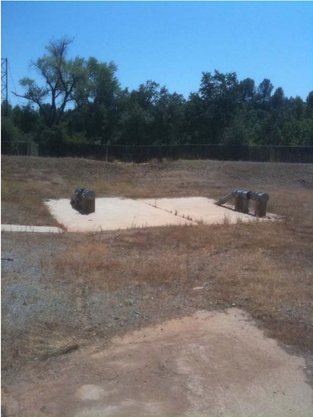
Photo 13: North Market lift station pipe taps and impoundment levy surrounding station shown in distance behind pipe taps.
