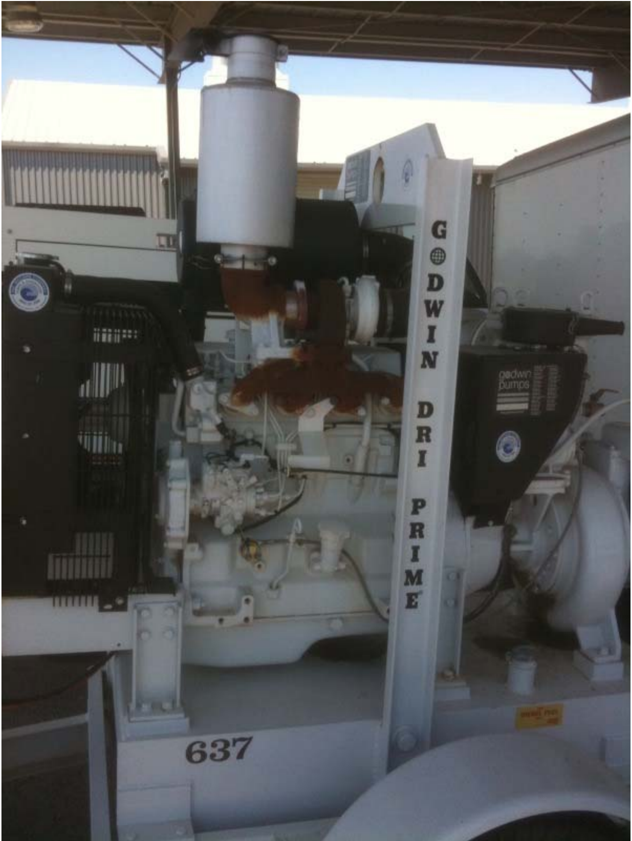
Photo 7: Trailer-mounted mobile emergency standby pump at City's Corporation Yard
