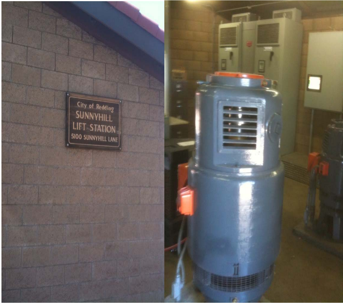
Photos 16-17: Sunnyhill lift station signage (L) and inspection of motors, pumps, and controls inside station (R)
