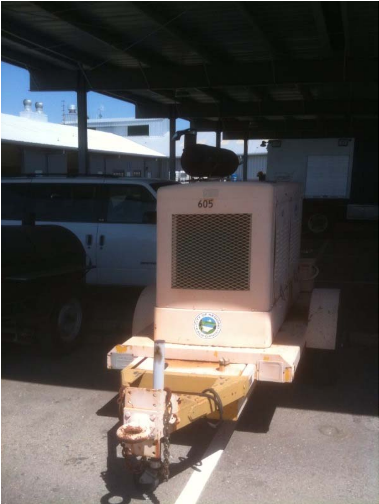
Photo 5: Trailer-mounted mobile emergency standby generator at City's Corporation Yard
