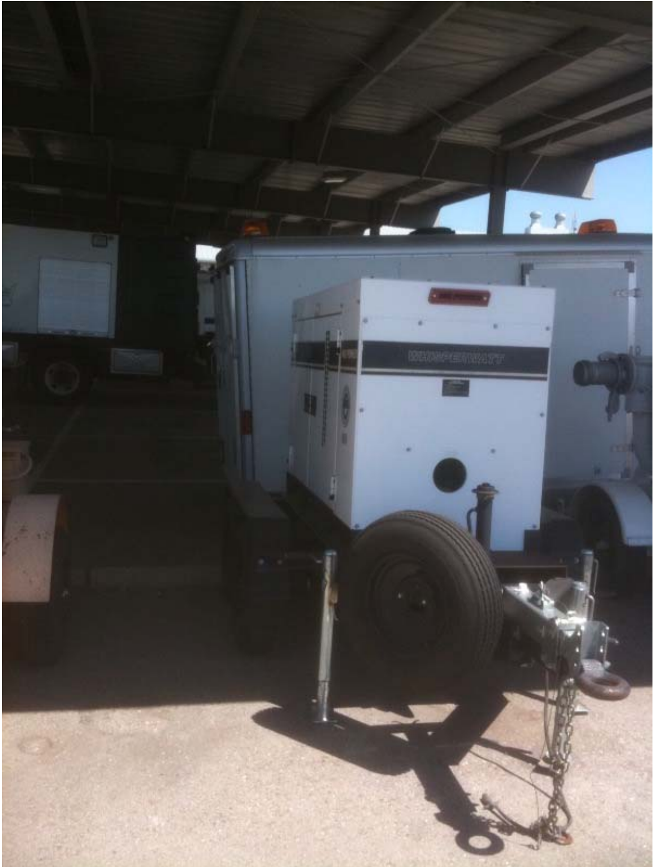
Photo 6: Trailer-mounted mobile emergency standby generator at City's Corporation Yard
