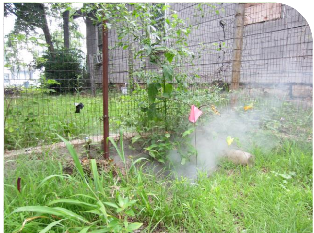
Smoke testing is used to detect sources of I/I. Image by Tetra Tech
