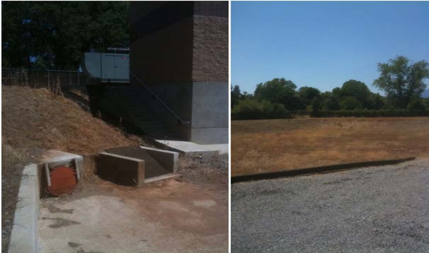
Photos 11-12: North Market lift station engineered impoundment gate valve and overflow drain (L), and impoundment levy (R)
