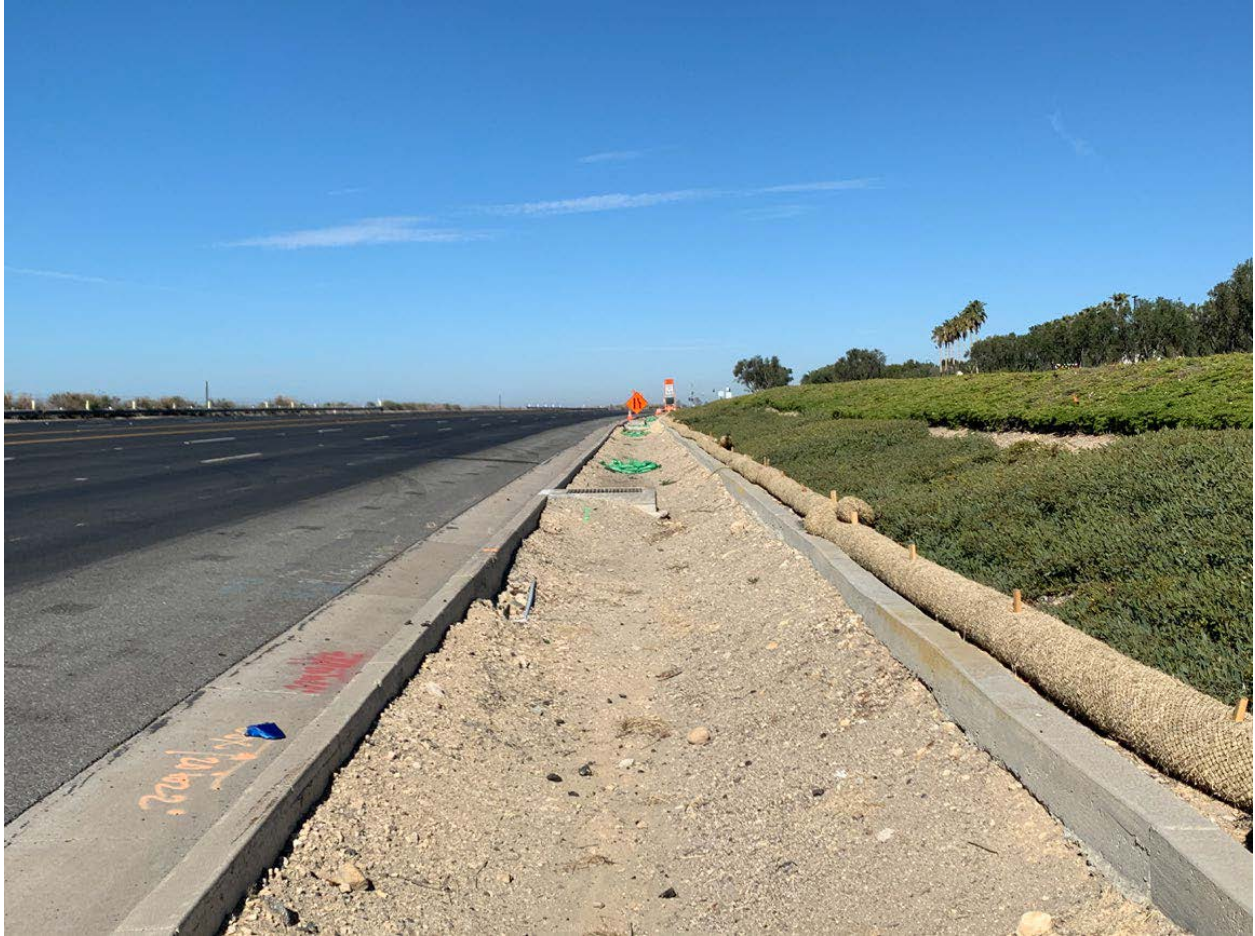
Figure E-6. Before 2/19/21
