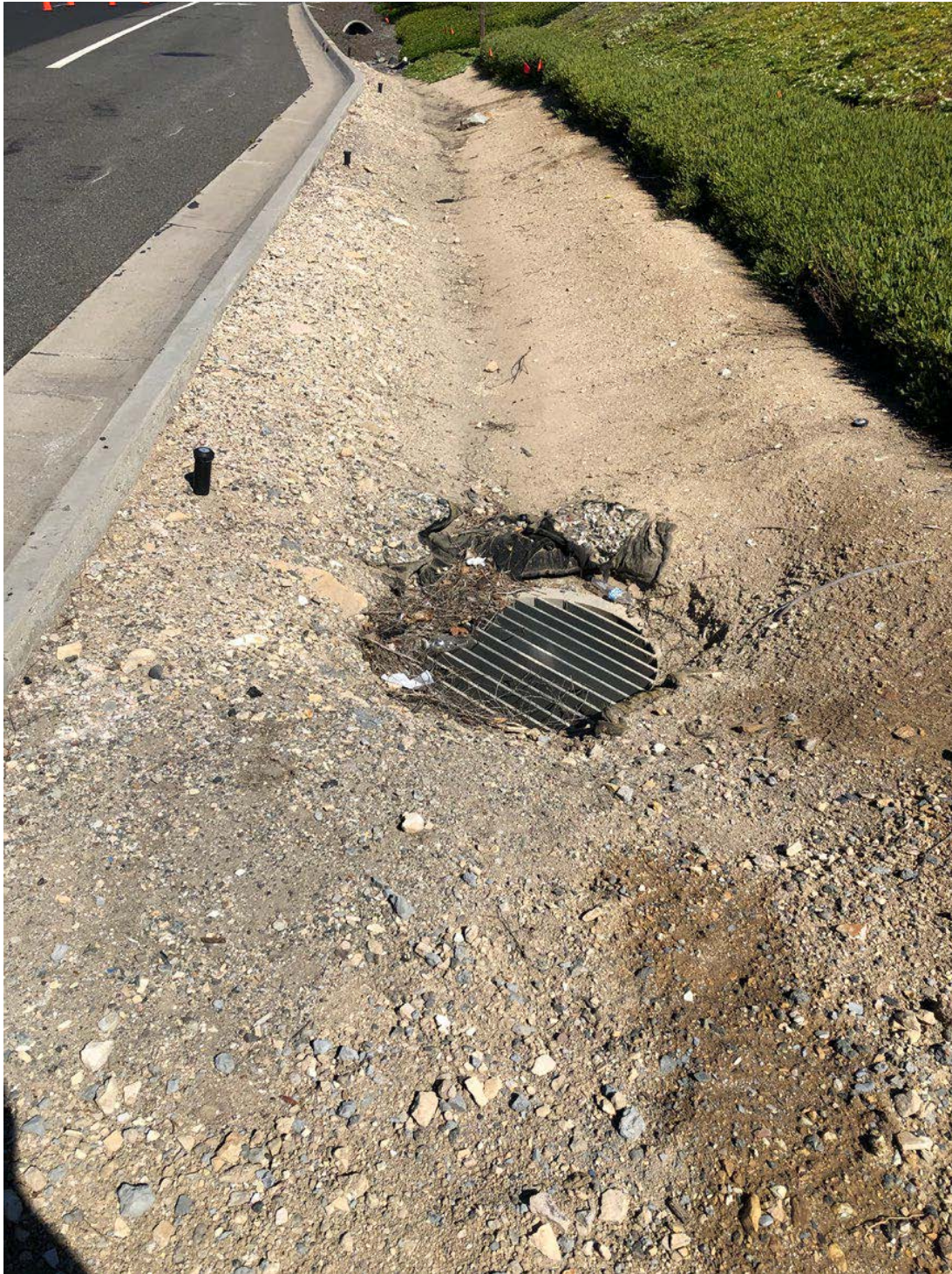
Figure E-1. Before 5/22/19
