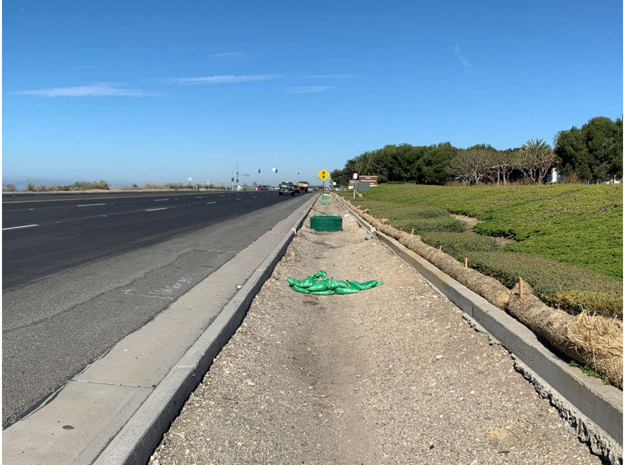
Figure E-2. Before 5/22/19
