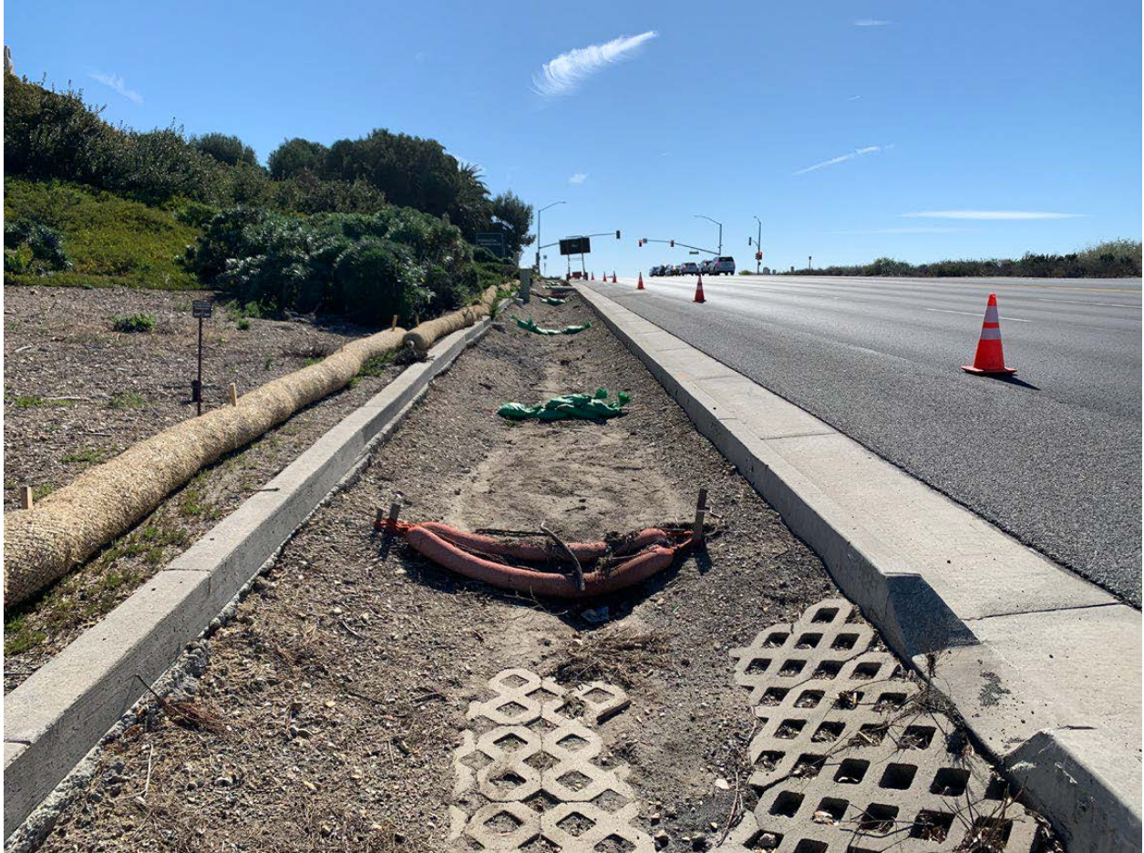
Figure E-3. Before 5/22/19
