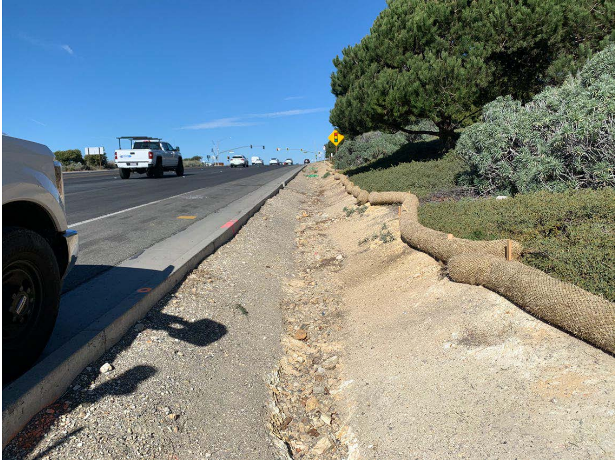
Figure E-5. Before 2/19/21
