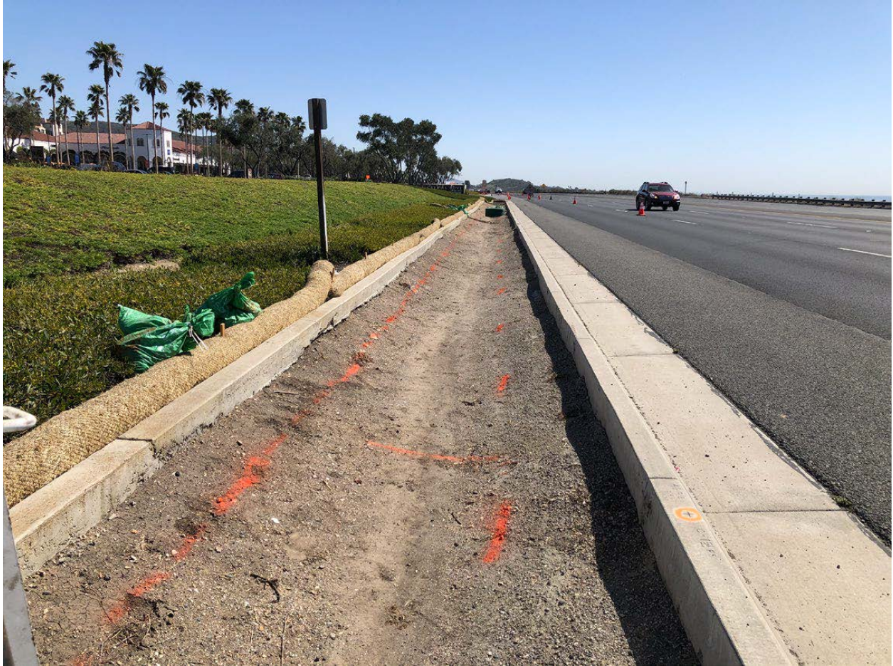
Figure E-4. Before 5/22/19
