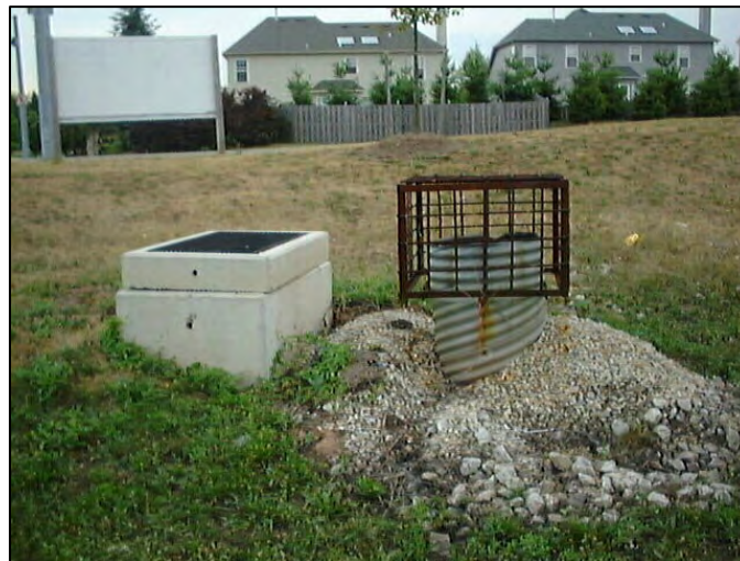
FIGURE 5-8 Sediment filter left in place after construction. SOURCE: Robert Traver, Villanova University.
