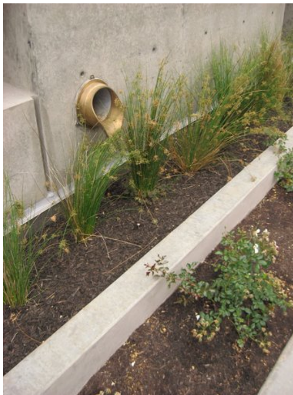
Figure 9. Disconnected downspout discharging to planter box.
