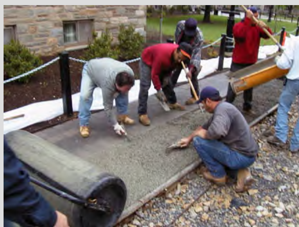
FIGURE 5-34 Infiltration bed under construction. Pervious concrete has functionality and workability similar to that of regular concrete. However, the pervious concrete mix lacks the sand and other fine particles found in regular concrete. This creates a significant amount of void space which allows water to flow relatively unobstructed through the concrete. This site was the first attempt at creating a pervious concrete SCM in the area, and there were construction and material problems. Since that time the industry has matured, and a second site on campus constructed in 2007 has not had any significant difficulties. SOURCE: Reprinted, with permission, from VUSP. Copyright by VUSP.
