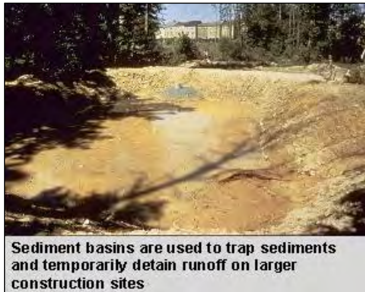
FIGURE 5-9 Sediment basin. SOURCE: EPA NPDES Menu of BMPs (available at http://cfpub.epa.gov/npdes/stormwater/menuofbmps/index.cfm?action=factsheet_results&view=specific&bmp=56 ).
