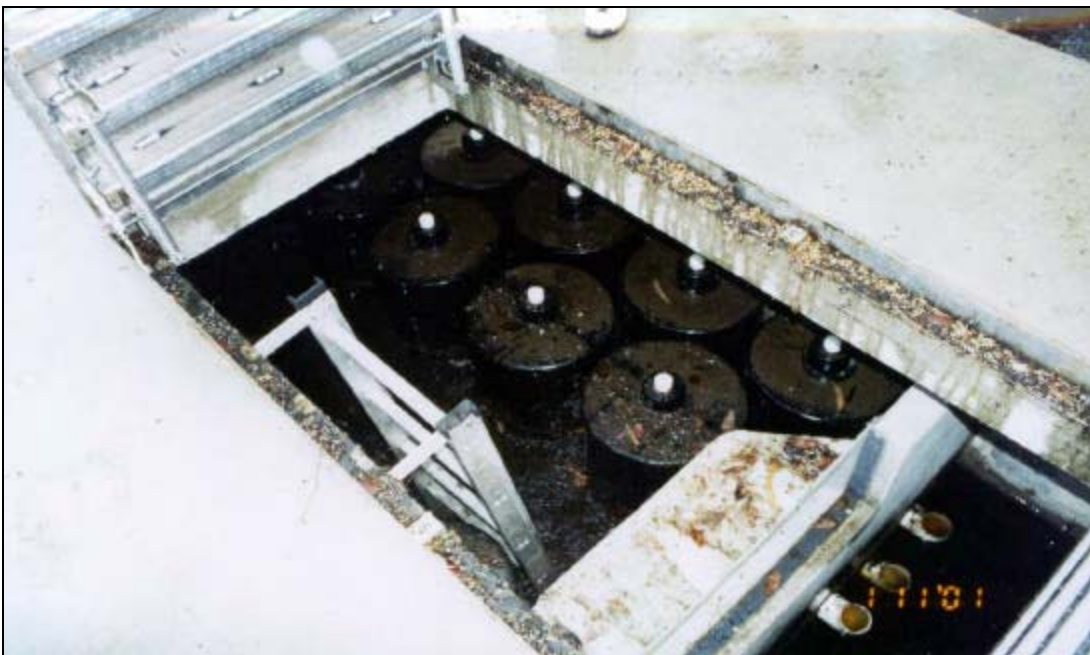
Figure 9-3 Internal View at Kearny Mesa
