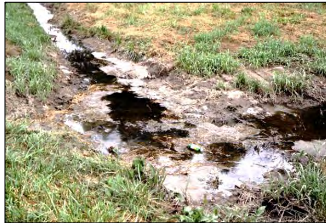
FIGURE 3-32 Failing sanitary sewer, causing upwelling of sewage through soil, and draining to gutter and then to storm drainage system. SOURCE: Robert Pitt, University of Alabama.
