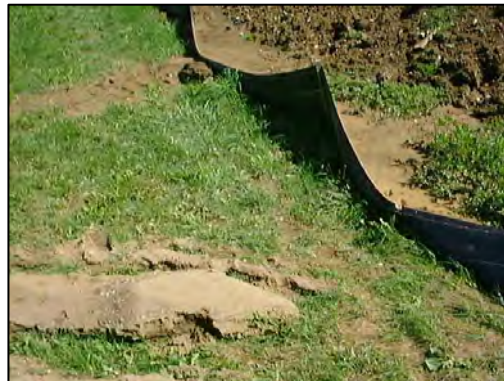
FIGURE 5-7 A functioning silt fence (top) and an improperly maintained silt fence (bottom). SOURCES: Top, EPA NPDES Menu of BMPs (available at http://cfpub.epa.gov/npdes/stormwater/menuofbmps/index.cfm?action=factsheet_results&view=specific&bmp=56 ) and, bottom, Robert Traver, Villanova University.
