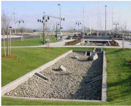
Figure 1. Media filter (City of Portland OR)
