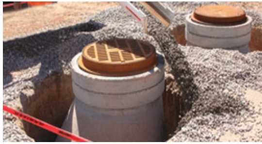
Figure 1. Dry well (Torrent Resources)
