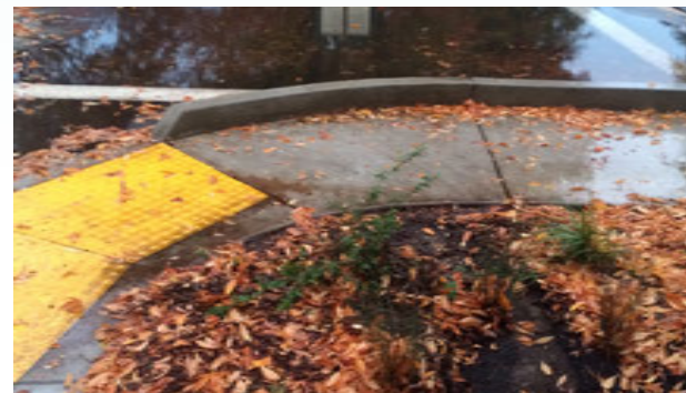
Sand and Sediment Entering SCM Drainage Area
