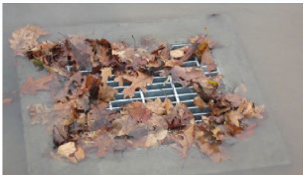
Leaf Debris Covering Overflow
