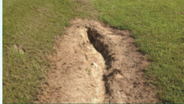
Erosion in Vegetated Swale (EPA 2016)
