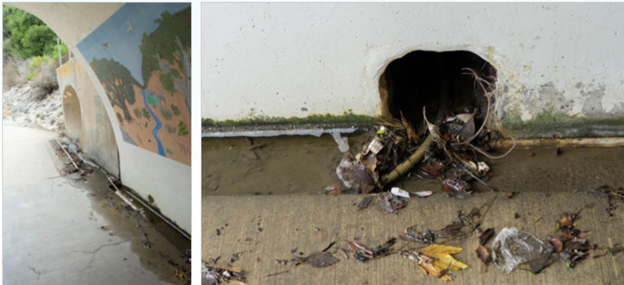
Figure IV-5. An outfall below a neighborhood and golf course discharging multiple pollutants.
