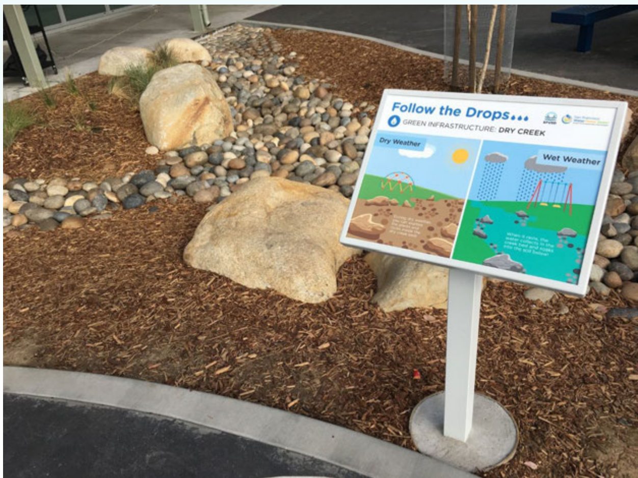
Figure I-11— Example of dry creek bed and signage installed at Robert Louis Stevenson Elementary School in San Francisco (SFUSD 2018)
