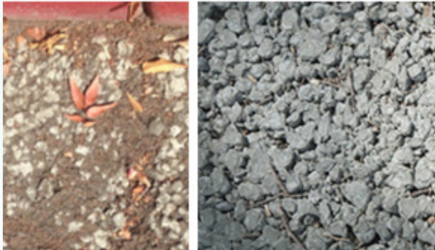
Porous/Pervious Pavement in Need of Maintenance vs. Clean
