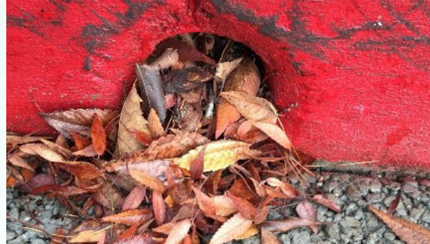
Leaves Clogging Inlet Pipe
