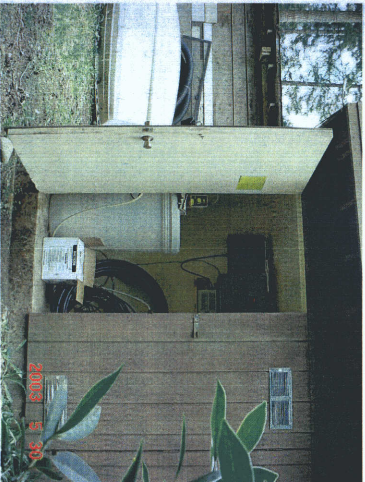
Chlorine injection and the pumping system are controlled from this shed near the POD.
