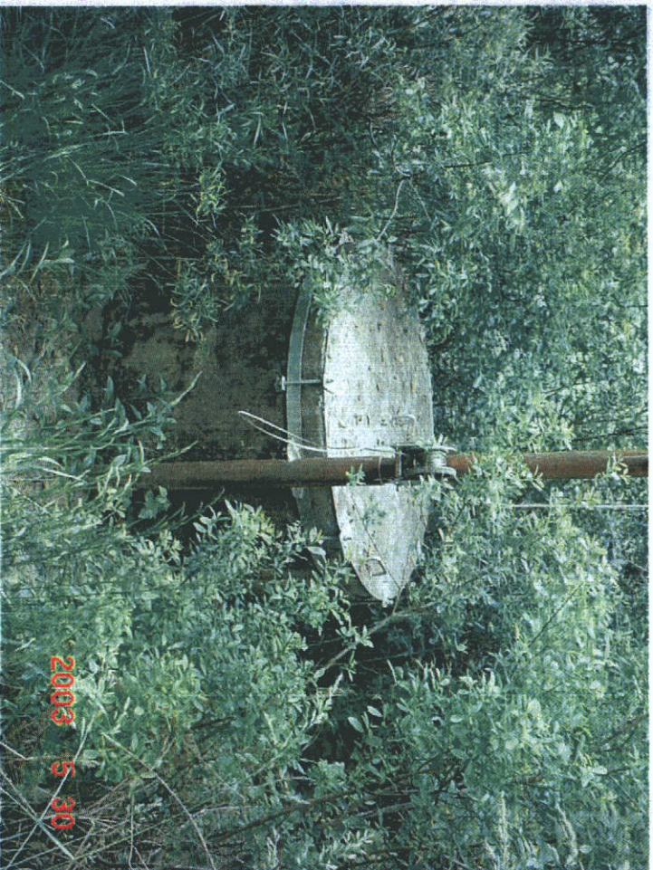
This is the sump for the Ranney collector. The pump is sealed in this concrete sump.
