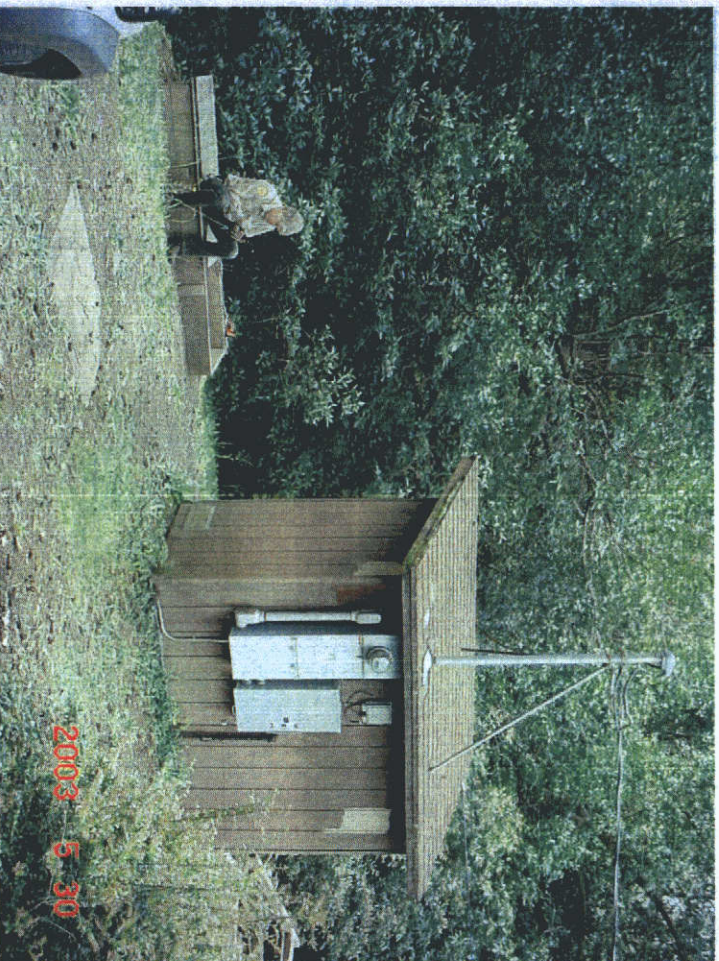
This view shows the electric meter on the rear of the control and treatment shed. The in ground vault on the left contains the water main section where chlorine is injected and the main meter.
