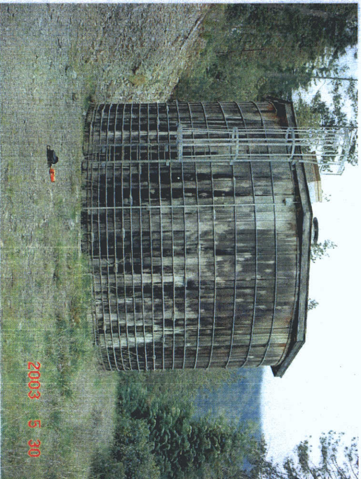
"Upper" storage tank with capacity of 50,000 gallons.
