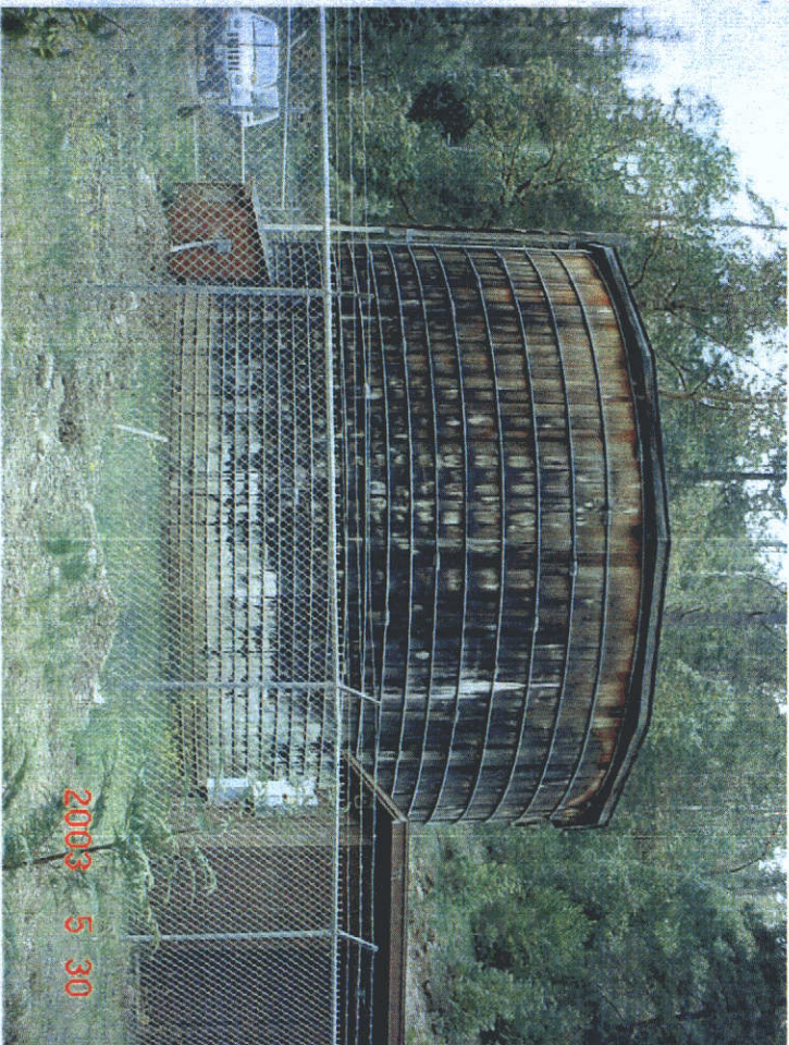
Primary storage tank with capacity 100,000 gallons.
