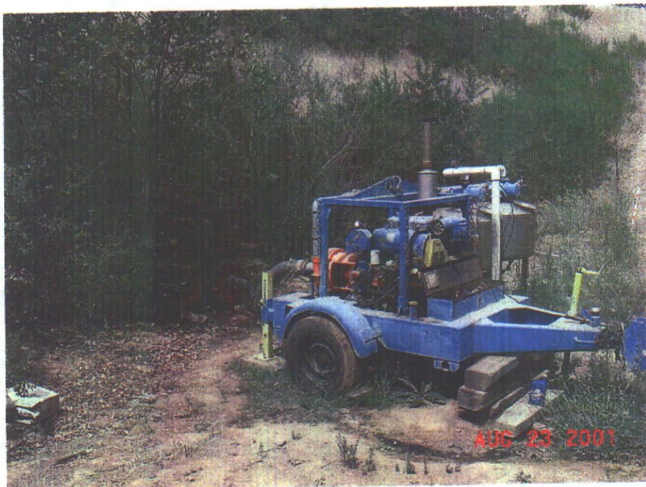
Pump at the toe of the Upper Reservoir dam.
