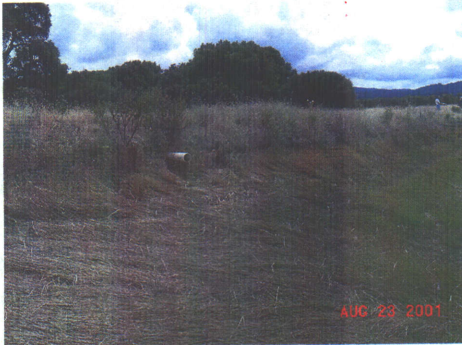
This photograph shows the spill pipe in the Upper Reservoir's dam on the day of the inspection.
