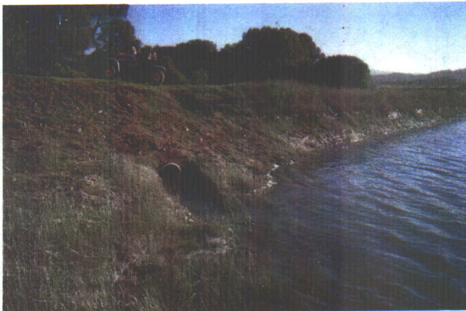
This photograph, taken after the inspection (about April 2002), was provided by the licensee and shows the spill pipe after it was lowered. The new elevation is not certain. Lowering it 4.5 feet from the inspected level would bring the capacity within compliance with the license. Lowering it 2.5 feet may only put the dam outside the jurisdiction of the Division of Safety of Dams.
