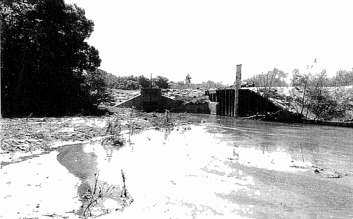
Point of Diversion #1 (Headgate to O'Neill Ditch)
