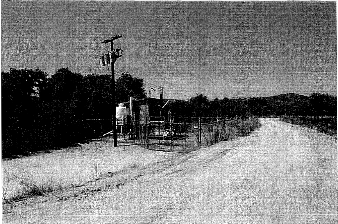
Point of Diversion #3 (Production Well Field) – Typical Well
