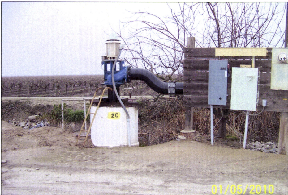
2.C. La Vina Ranch Pump Point of Rediversion on Cottonwood Creek
