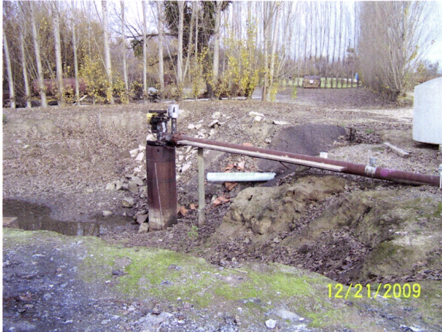
6. Rancho Bella Vista Pump Point of Rediversion on Fresno River at River Mile 23.5
