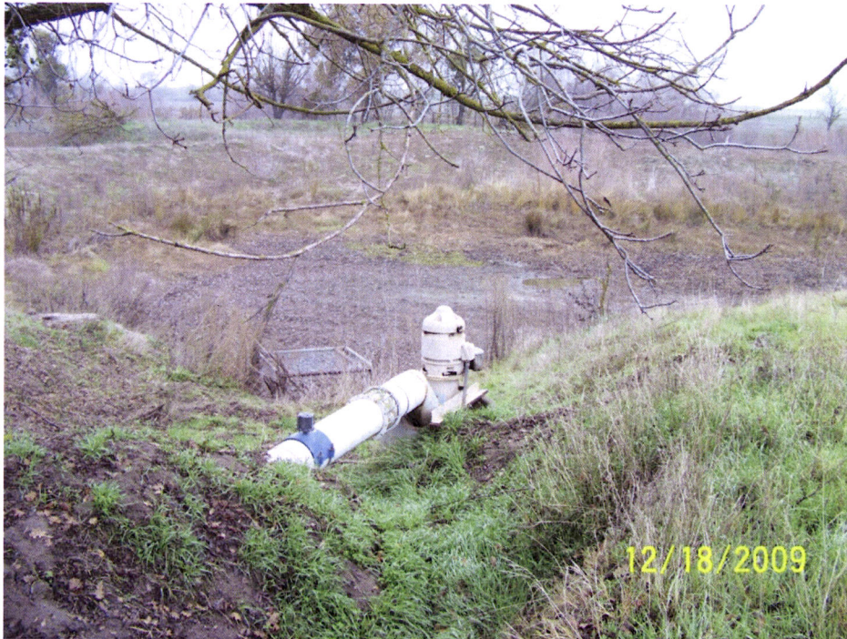
1. Adobe Ranch Pump Point of Rediversion on Fresno River at River Mile 28.4 North 1,840,670 feet and East 6,726,220 feet, being within SW¼ of NE¼ of Section 19, T10S, R19E, MDB&M.
