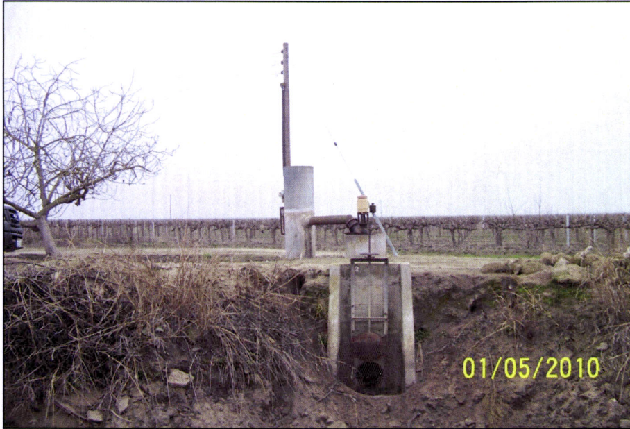
2. Cavaletto Pump Point of Rediversion on Cottonwood Creek
