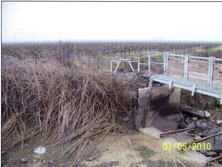
13. Galeener Ditch Diversion Dam Point of Rediversion on Cottonwood Creek
