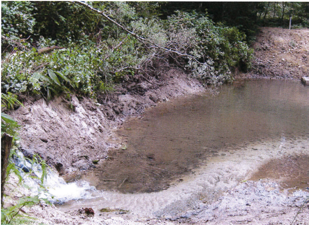
Point of Diversion at Waterfall Gulch Looking Downstream – Intake at Upper Right (July 30, 2013)
