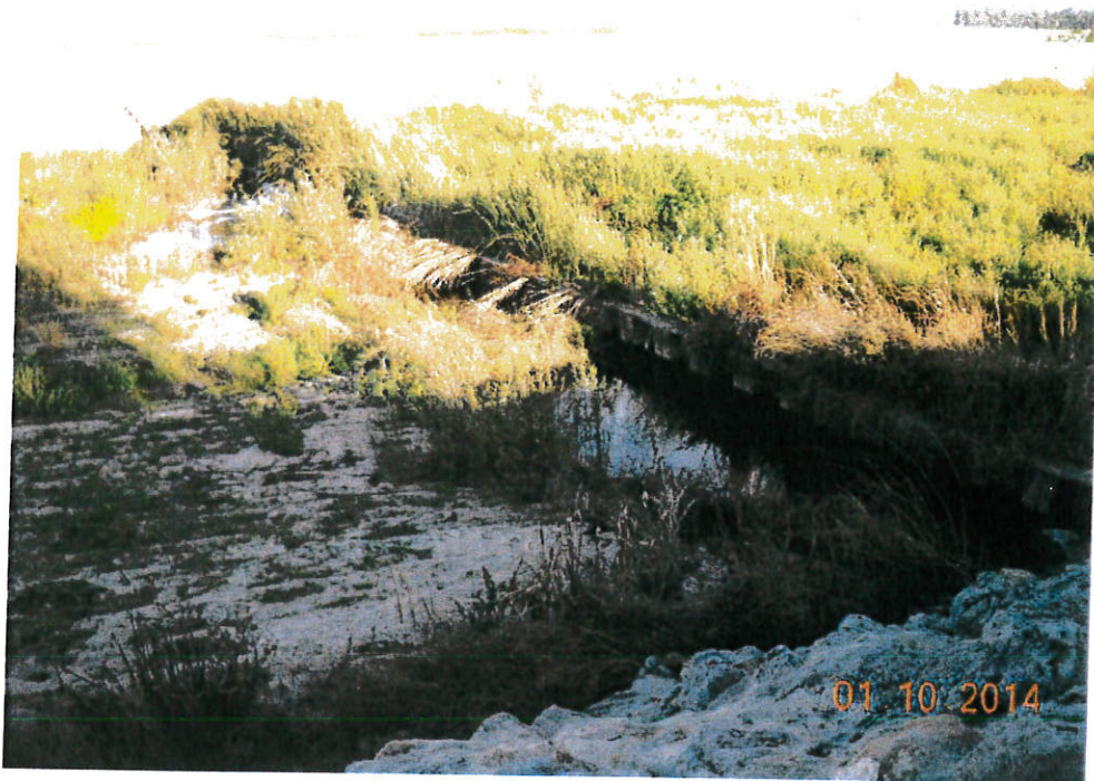
Photo 21. Calleguas Creek downstream of the Old Lewis Road Bridge showing grade control structure that is a fish migration impediment
