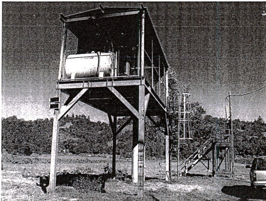
Point of Diversion #1 – Russian River Pump
