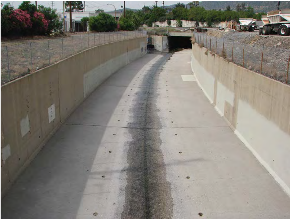
PHOTOGRAPH 2. Concrete-lined rectangular open channel upstream of Discharge Point 002 looking upstream toward the northwest.
