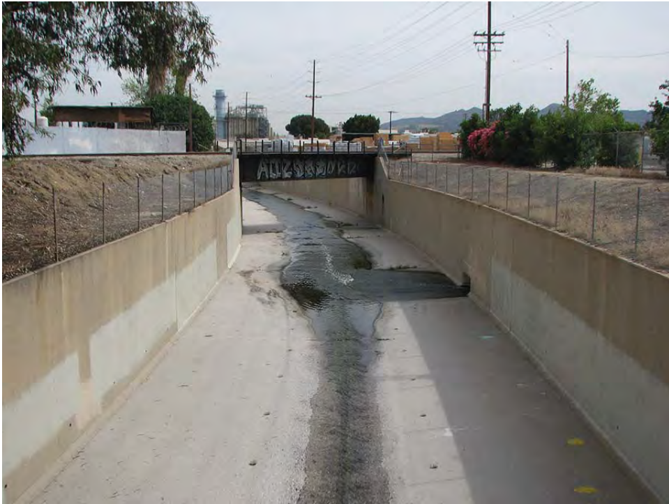
PHOTOGRAPH 1. BWRP Discharge Point 002 into a concrete-lined rectangular open channel looking downstream to the southeast.
